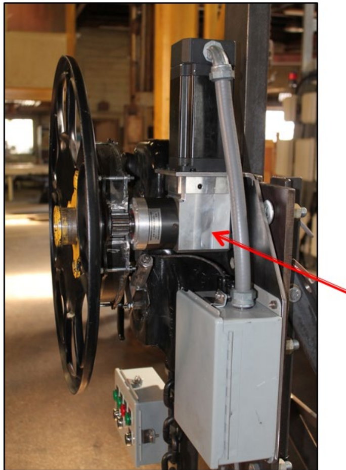
Figure 5 – New Gearbox Installed in New System
