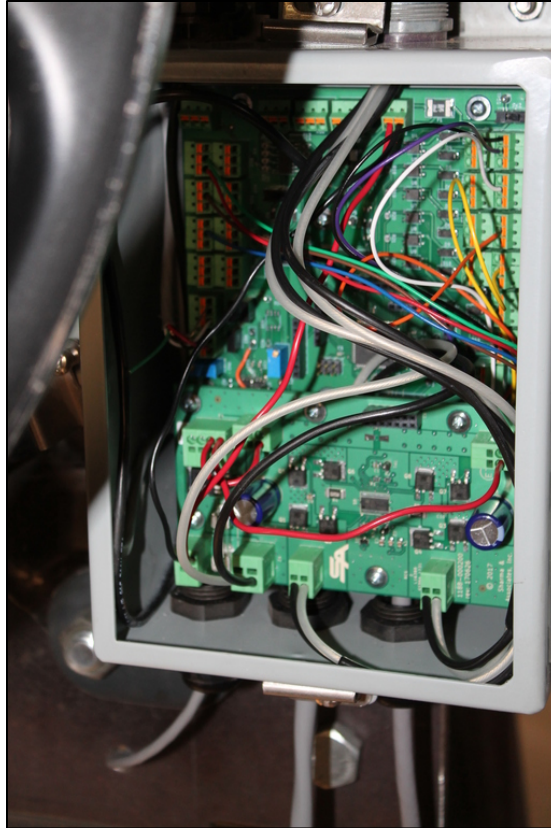
Figure 7 – Redesigned Controller Installed in the EDHB Control Box
