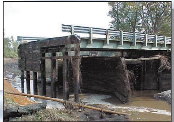
Some bridges were so severely damaged that they had to be replaced.
