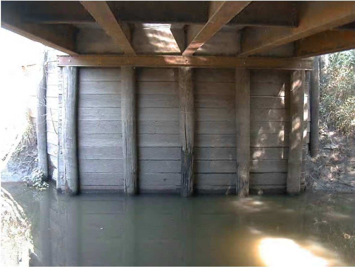
Figure 7.2. KCB2 Pile Deterioration.
