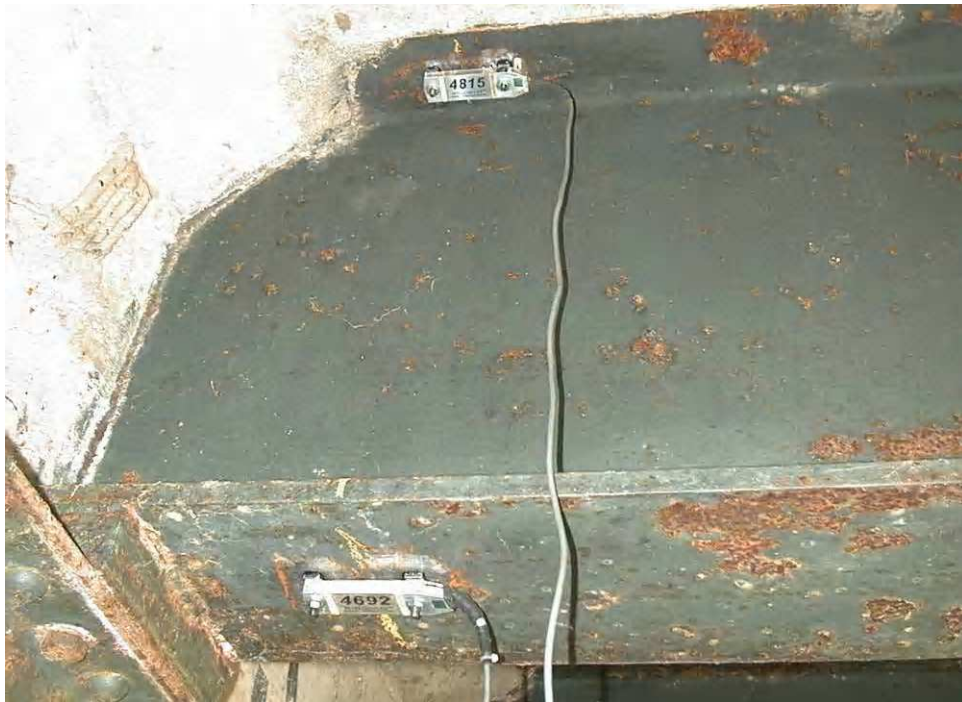
Figure 4.8. Instrumentation Near Abutment of MCB.
