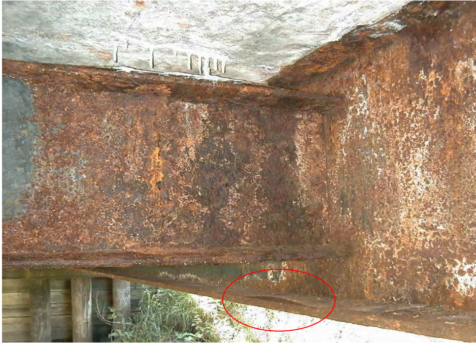
Figure 4.2. MCB Girder 2 Deterioration and Delamination.
