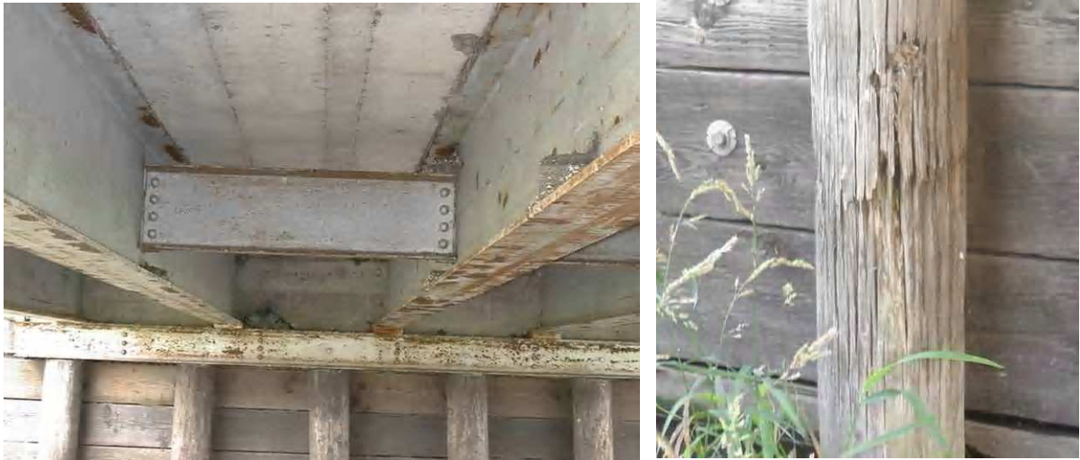
(a) Minor rust on girders
