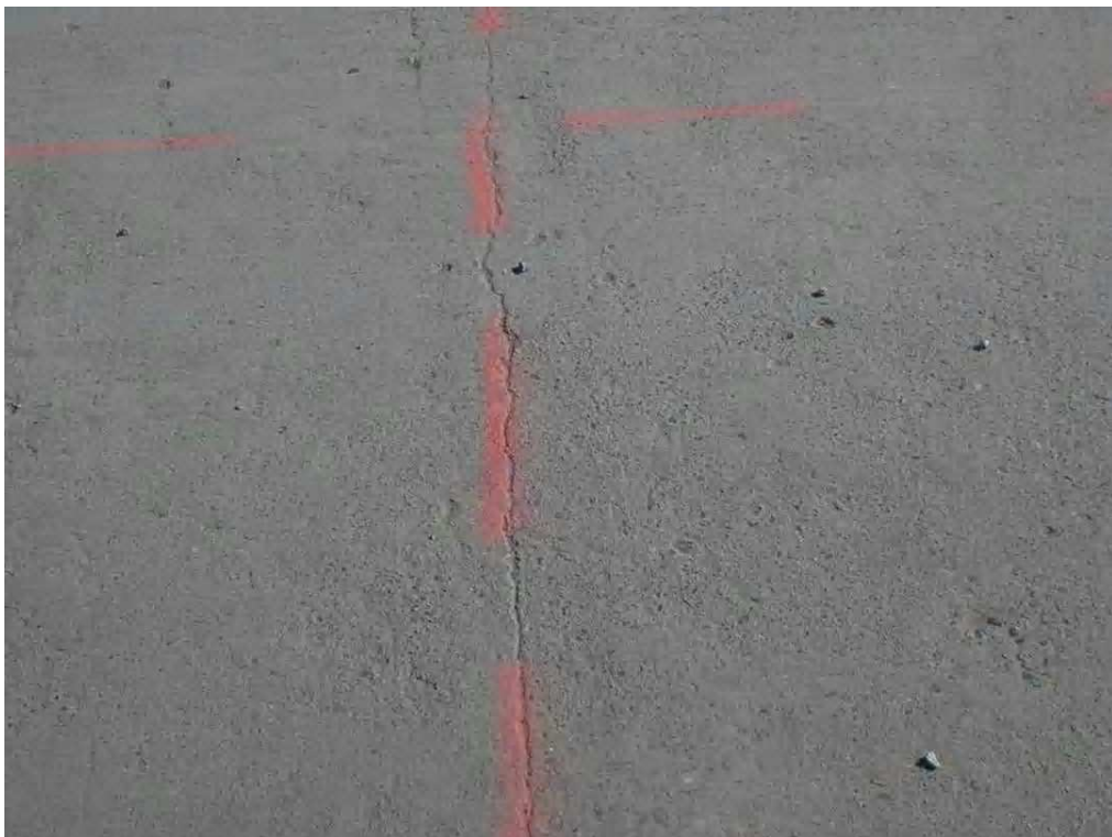
Figure 5.3. KCB1 Deck Crack.
