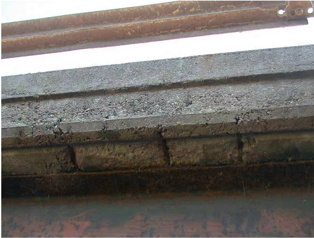
Figure 5.2. KCB1 Poor Concrete Consolidation.
