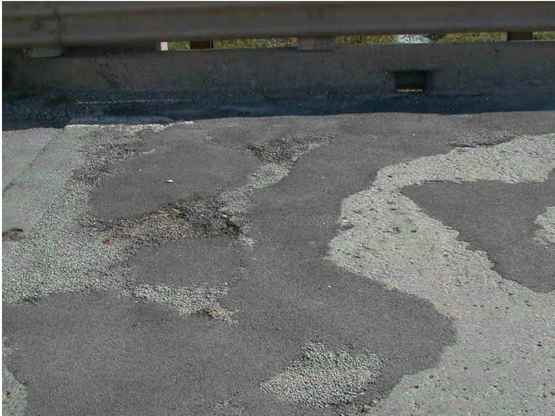
Figure 6.2. Asphalt Patches in CCB Concrete Deck.
