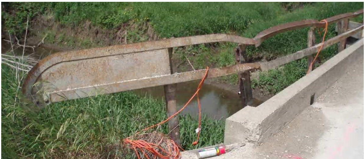
Figure 7.3. KCB2 Railing Damage.
