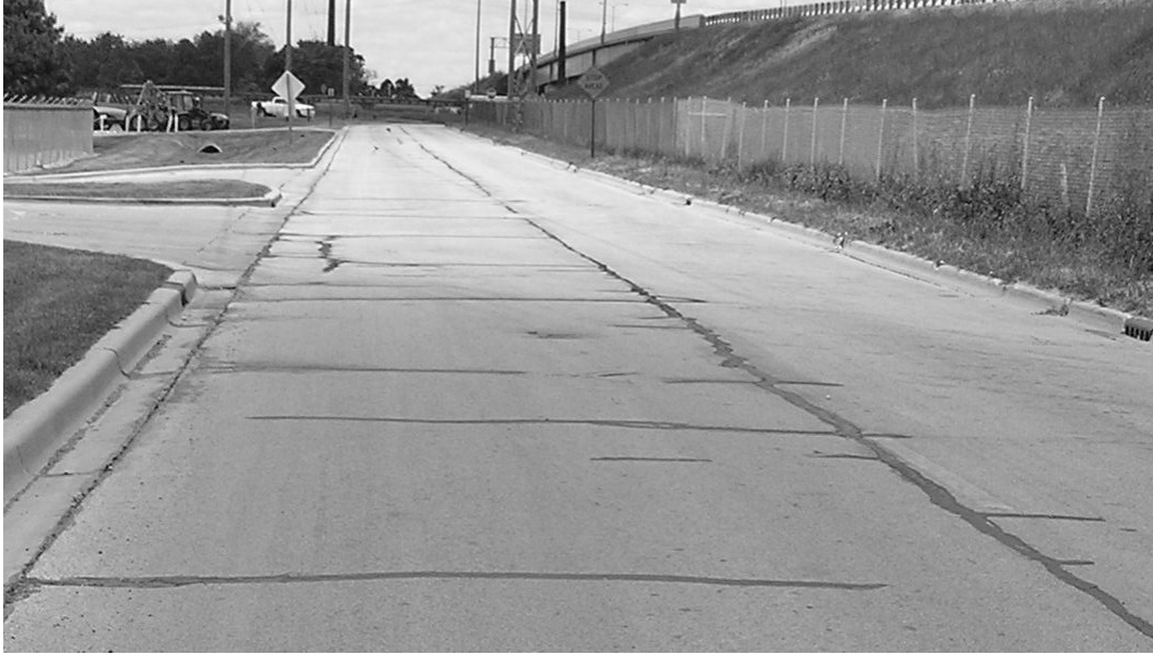
Figure 8.1. Observation of an asphalt overlay bonded to a base-layer with uniformly distributed cracks due to low temperature loading
