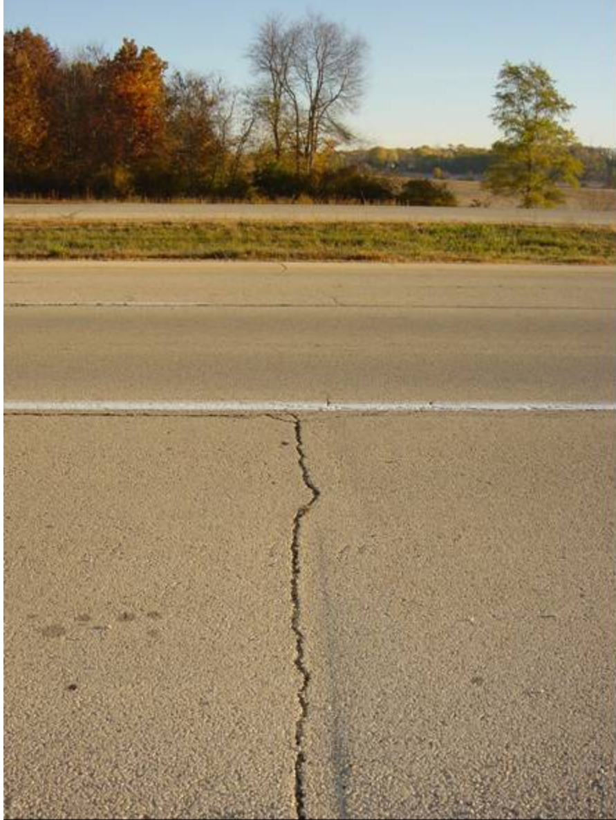
Figure E-2. Shoulder cracking
