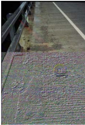
Figure 8.5-1 - Scaling along the curbline. This is due to excessive hand-finishing and over-working the concrete prior to curing.
