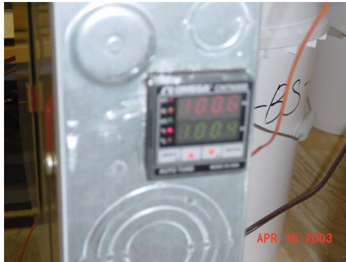
(b) Thermostat with power control
