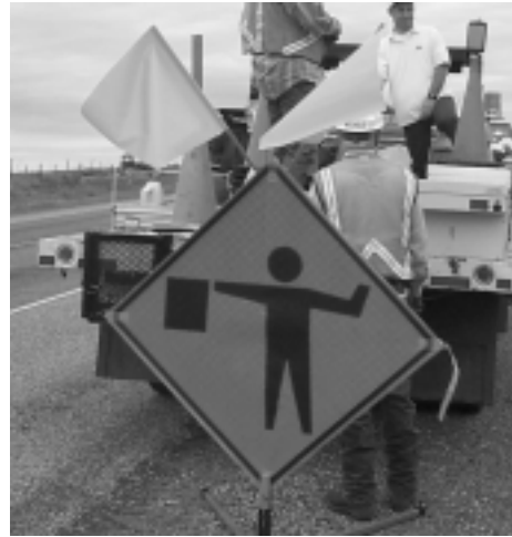
Fluorescent Orange Sign.
