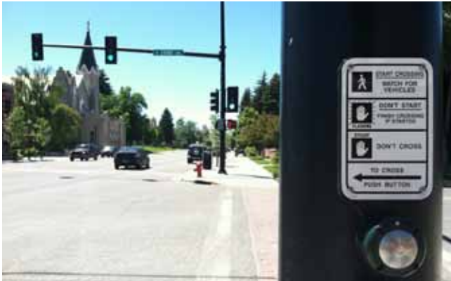
If pedestrian volumes are high, push buttons are not needed.; these push buttons in Bozeman were deactivated for daytime use
