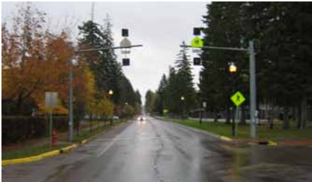
Pedestrian actuated flashing beacon in Whitefish
