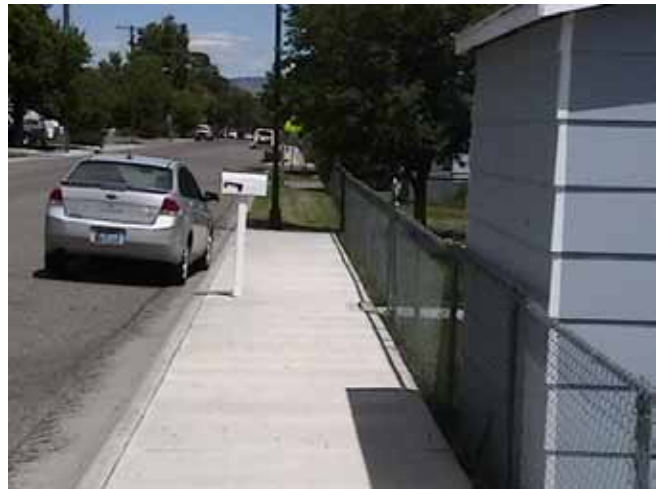
Missing section of sidewalk in Livingston
