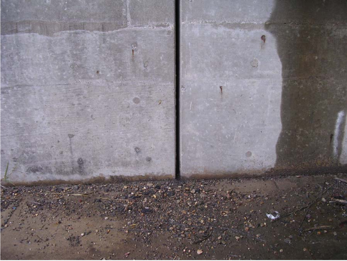
Figure 3.16: Signs of Soil Infiltration Between Panels N-3 and N-4
