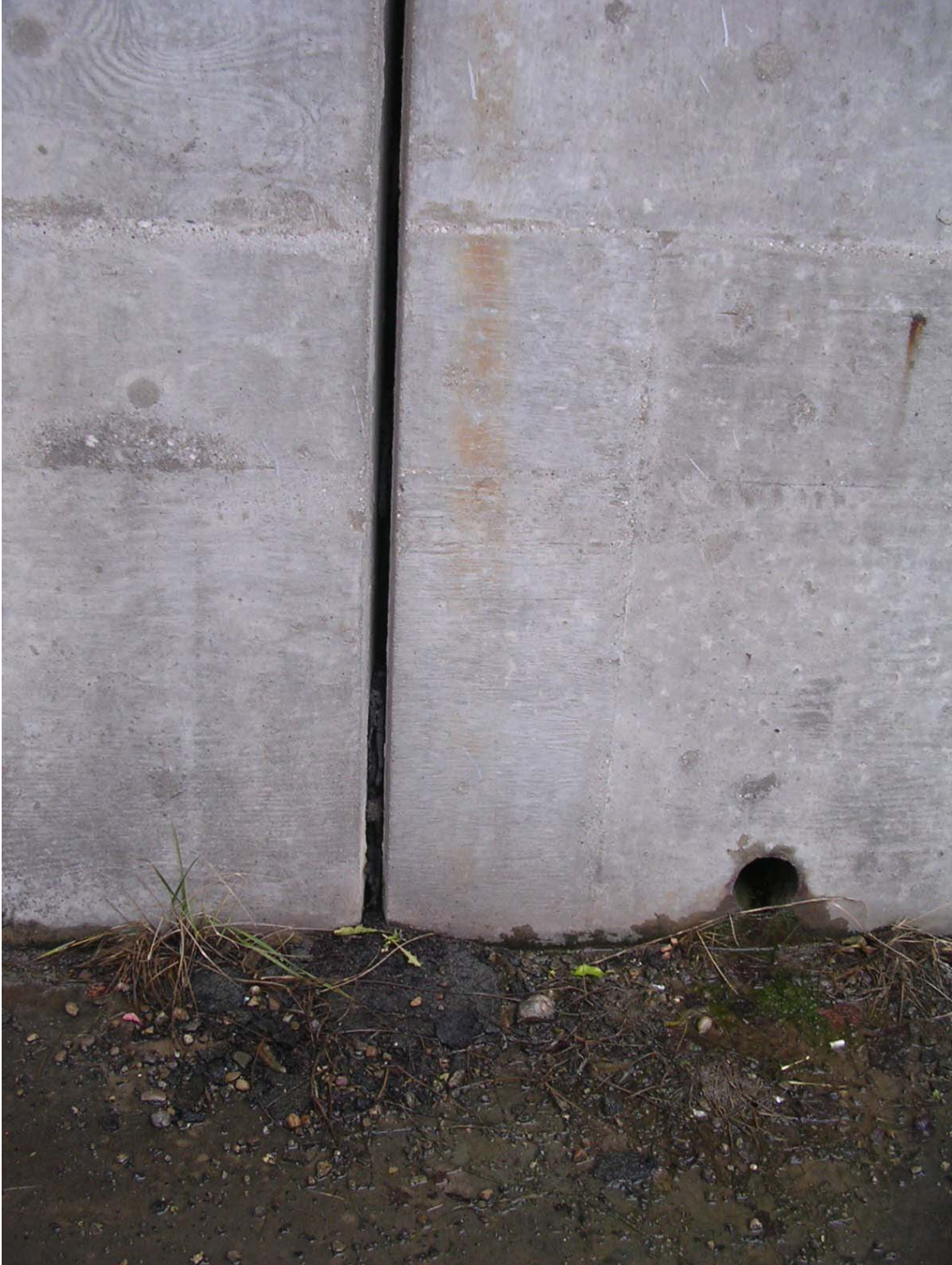
Figure 3.14: Signs of Soil Infiltration Between Panels N-2 and N-3
