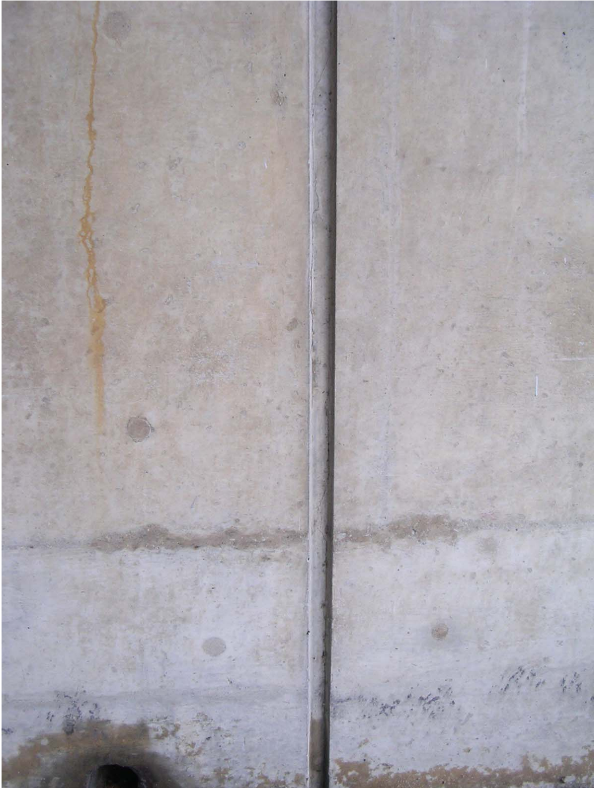
Figure 3.21: General View of Panel N-5 (Photo C)
