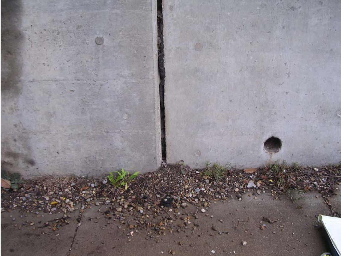
Figure 3.22: Signs of Soil Infiltration Between Panel N-5 and NE Wingwall
