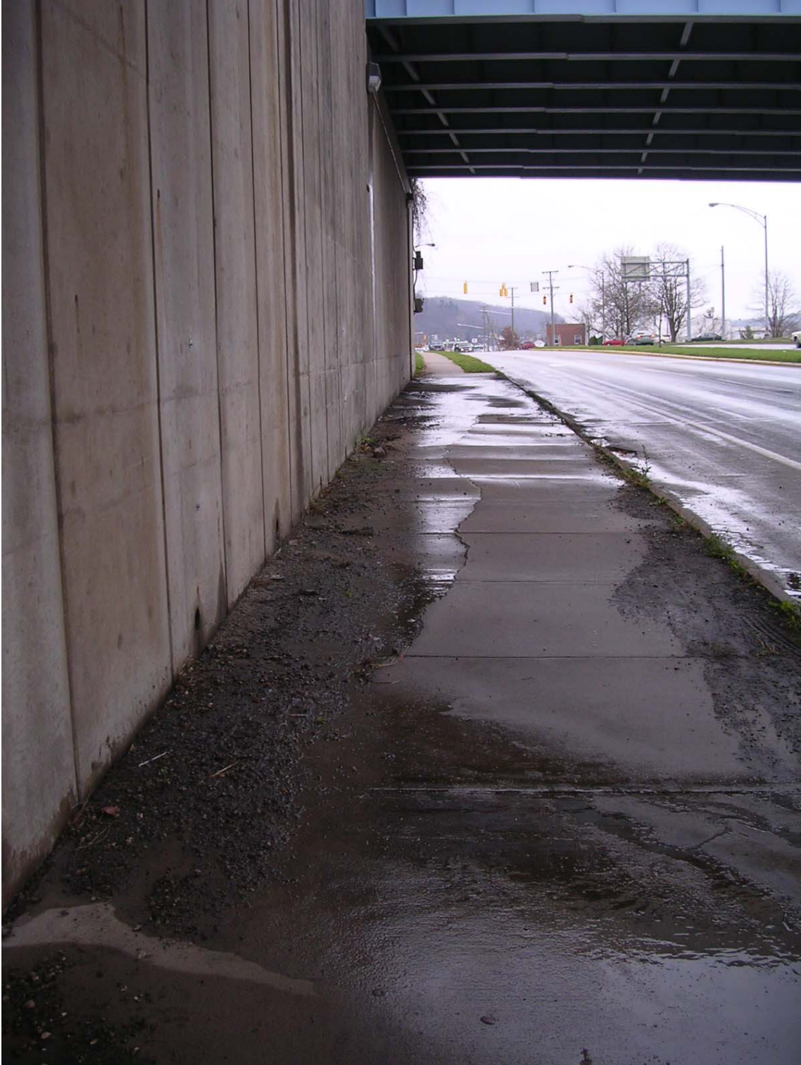
Figure 3.11: Cracked Sidewalk on North Side of E. State St.
