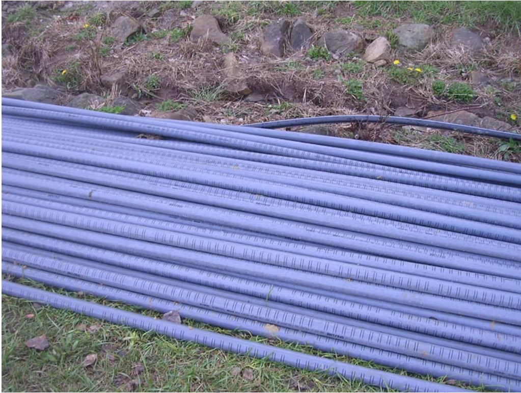
Figure 3.27: PVC Pipes Used as Horizontal Drains
