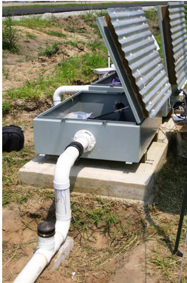
Figure 5.7 – Data Acquisition Enclosures
