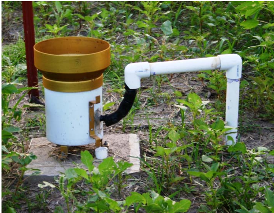
Figure 4.25 – Installed Tipping Bucket
