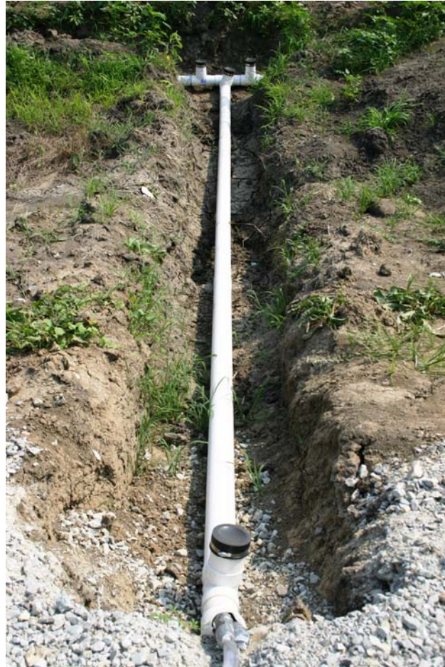
Figure 5.8 – Lateral Pipe Extending From the Shoulder to the Header
