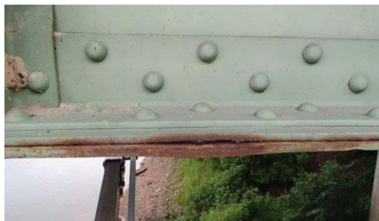
Figure 4.16 Pack rust in the edges of the splices (location 3).
