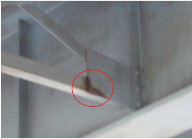
Figure 4.10 Example of pack rust in cross bracing.
