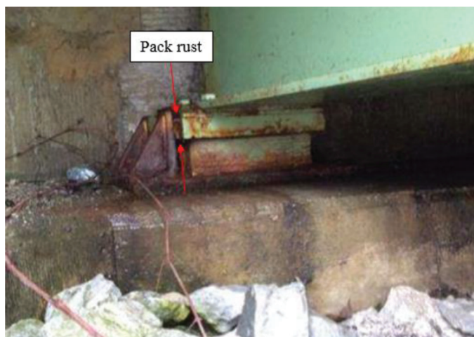
Figure 4.18 Pack rust in elastomeric bearings.
