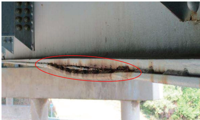
Figure 4.9 Non-continuous welds between the cover plate and bottom flange (location 3).
