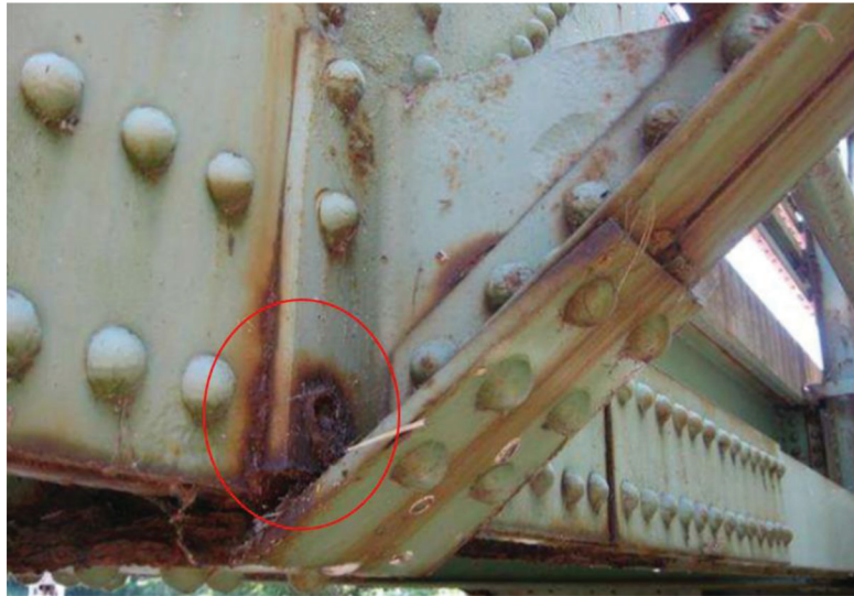
Figure 4.3 Rivet failed due to pack rust.
