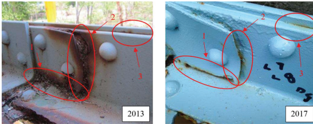
Figure 4.5 Pack rust in connections of the bottom chord.
