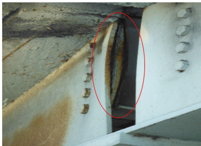
Figure 4.2 Most severe pack rust in the diaphragm found in Indiana.
