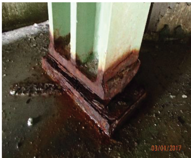
Figure 4.17 Pack rust in the rocker bearings.
