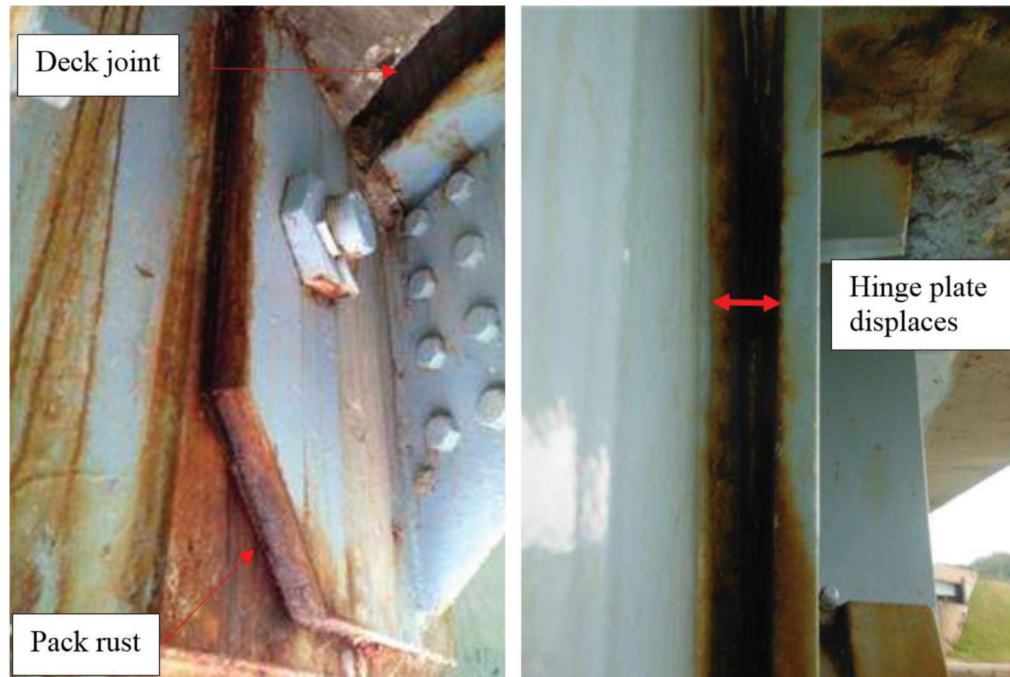
Figure 4.13 Pack rust in the hinge-pin connection.
