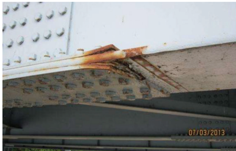
Figure 4.15 Pack rust in the corners of the splice plate (location 2).
