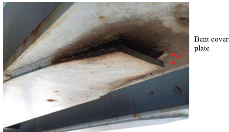
Figure 4.8 Pack rust at the end of the cover plate (location 2).
