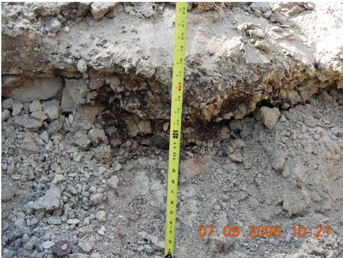
Figure A1 . Organic-Rich Zone in Subgrade Soil.
