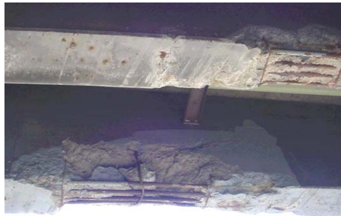
Fig. 1. Impact damages in the concrete bridge girders by over-height trucks
