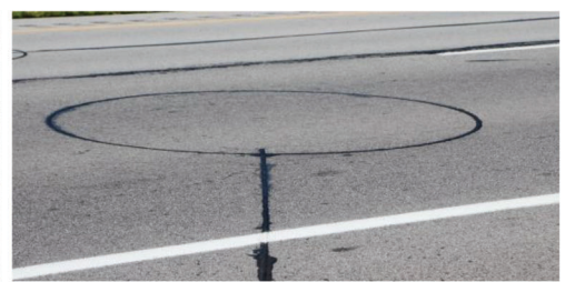
(c) Inductance loop at WIM station
