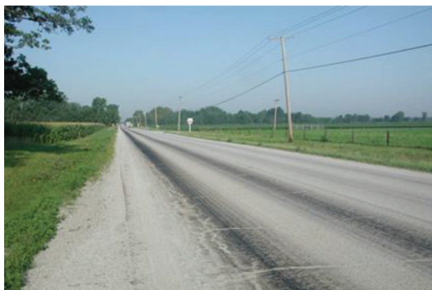
Figure 2.1 Photo of chip seal experiencing aggregate loss.
