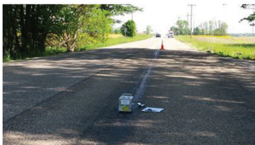
(a) Bleeding occurred in left wheel path
