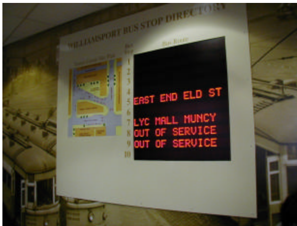
Variable message signs show buses in the terminal and their bus bay locations.
