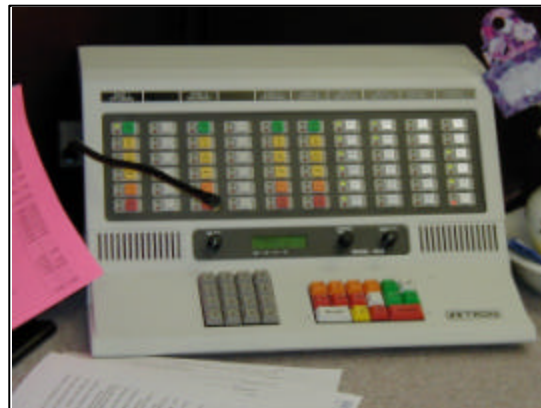
This Motorola base station is part of the communications system procured by OTA in their rural ITS deployment.
