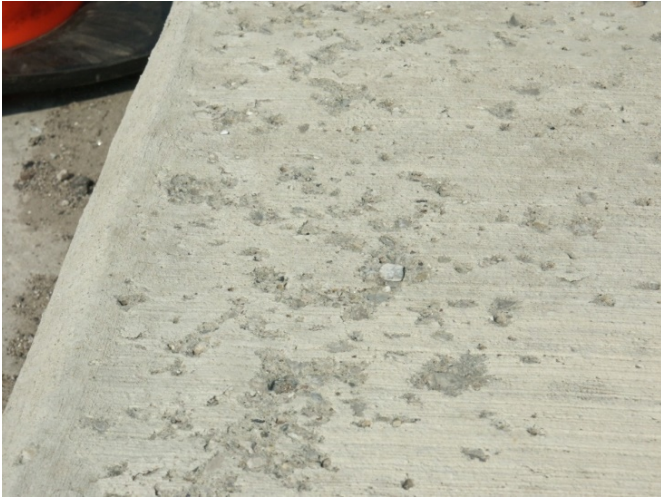
Figure 2. Concrete surface suffering deicer scaling. (source: Tom Van Dam)
