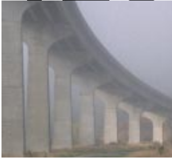
PONTIS 2000, a Windows®-based bridge management software tool developed by FHWA, analyzes cost and condition data of bridge components for long-term preservation and improvement.
