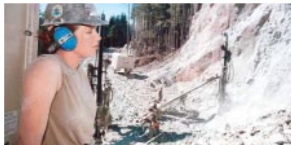
Drilling rock on Annette Island, Alaska, part of the $33 million project to link the remote island to the mainland. Innovative applications included geodesic construction technology developed and pioneered by FHWA. Photo courtesy of: DoD
