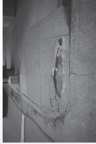
Figure 10-2. Sidewalk cracks and broken concrete are common sidewalk maintenance problems that inhibit pedestrian access to sidewalks.
