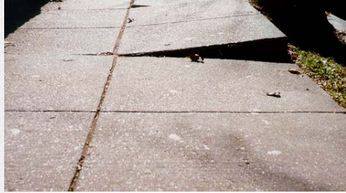
Figure 4-36. Changes of level in sidewalks caused by tree roots are potentially hazardous for pedestrians.
