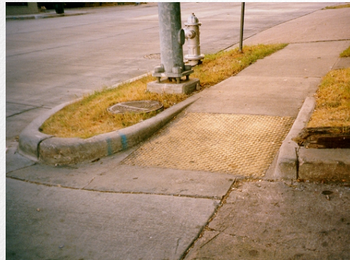
Figure 7-18. Detectable warnings at the bottom of curb ramps enhance access for people with vision impairments (Austin, Texas).
