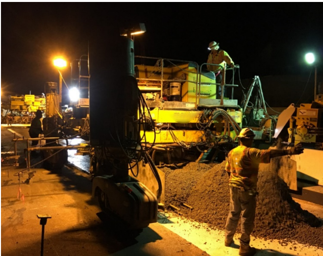
© Applied Pavement Technology 2017
