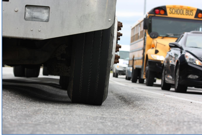
Figure 2. Photo. Deep rutting in the AC pavement at the intersection stop line.
