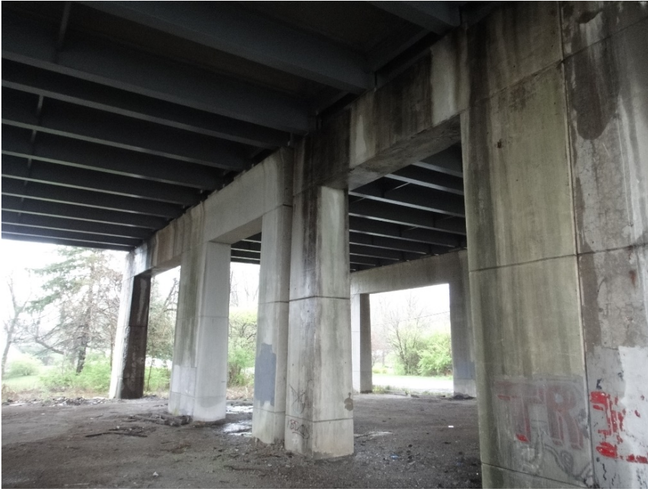
Figure 1. Deteriorated concrete columns and pier cap under leaking joint.
