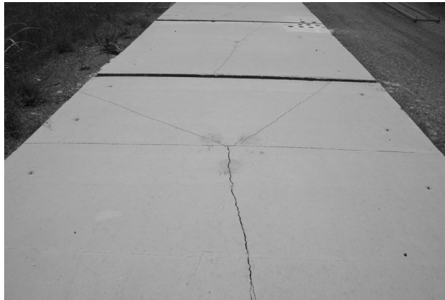
(a) Plan view of the failed slabs
