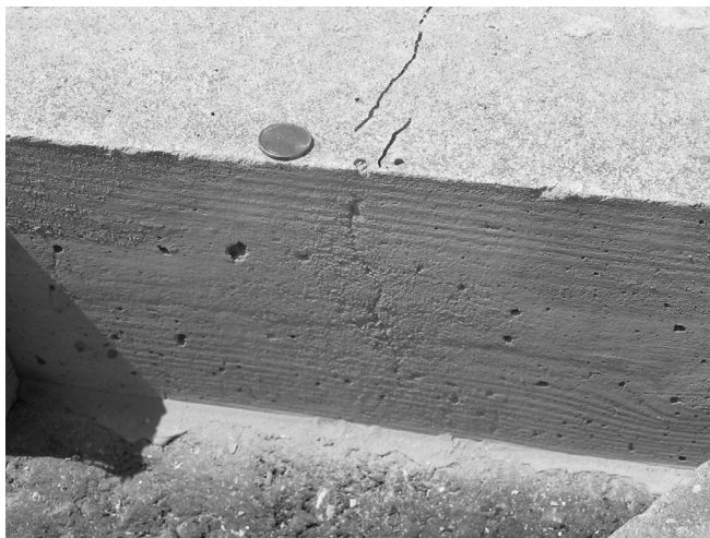
(c) Partial-depth edge crack after fatigue failure
