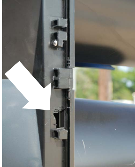
Figure 6-3. Failure at connection for the backplate on polycarbonate signal (Test 22) (Photo courtesy of author)
