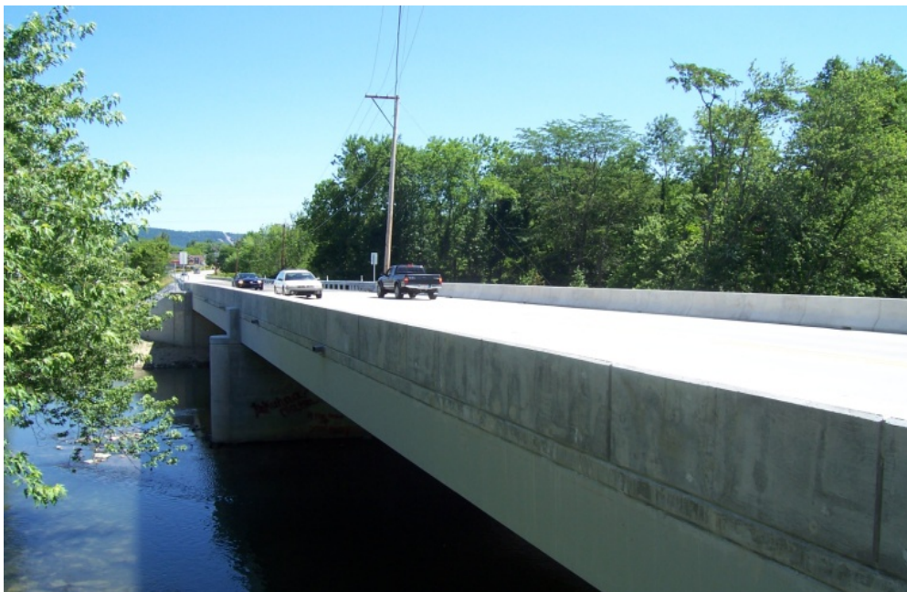
Route 34 Bridge – Carlisle, PA (ARRA Funded Project). Recently recognized as the “Best Recovery Act Project” in the small project category as part of the America’s Transportation Awards program sponsored by AASHTO.
