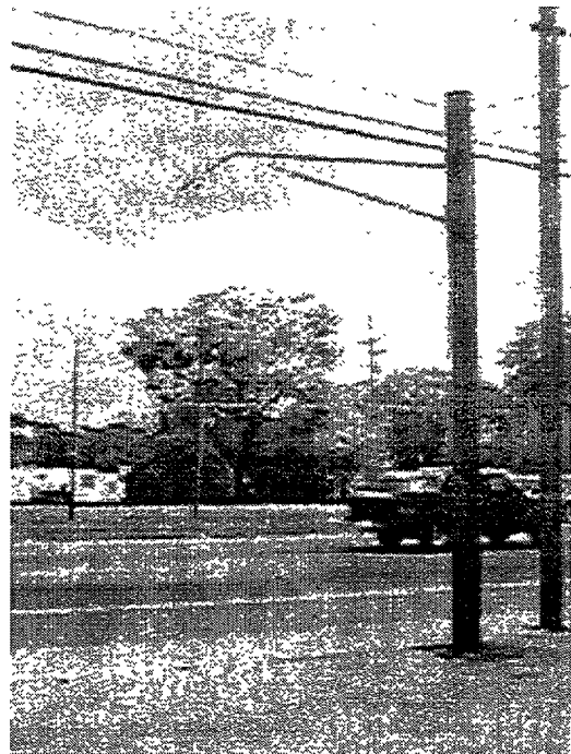
FIGURE 9 VDAC mounted on mast arm.
