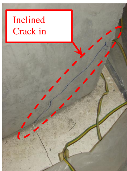
Figure 6-38: Footing Failure in Specimen CSR
