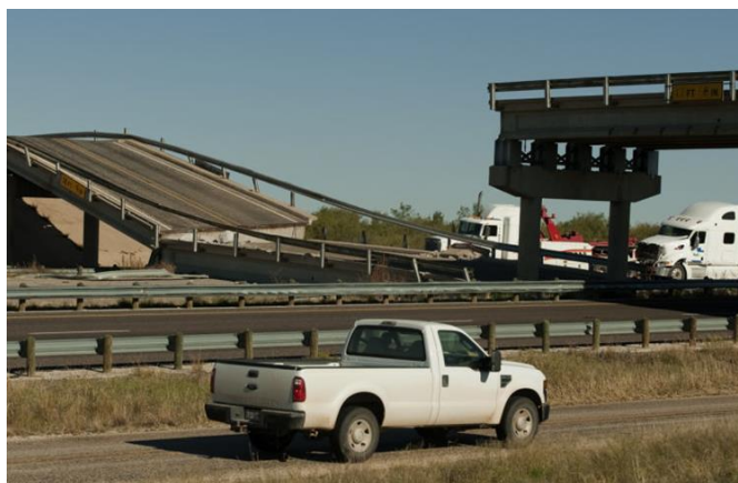
Figure 6-3: I-80 Bridge Collapse near Big Springs, TX (Midland Reporter Telegram, 2013)
