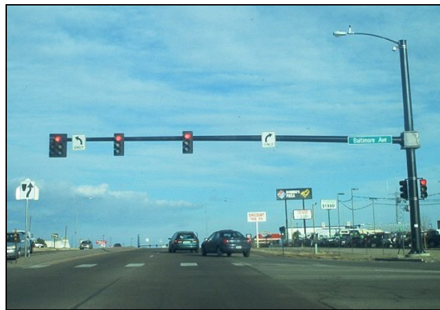
Figure 1.2. CDOT specified high-speed intersection traffic signal (Salek, 2006)
