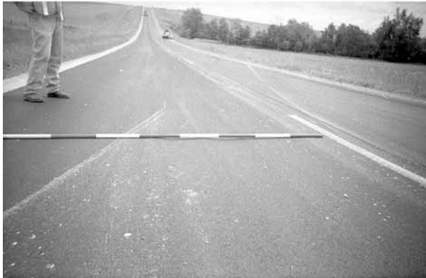
Rutting in the newly-placed first lift.
