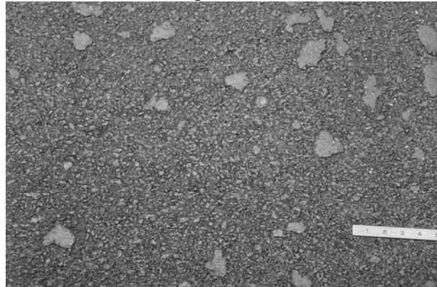
"Patties of AC on pavement surface due to inadequate roller tire temperature.
