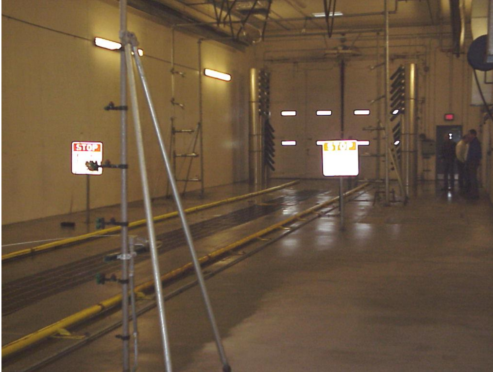
Figure 4.1: Dedicated Snow Plow Washing Facility, Minnesota DOT.
