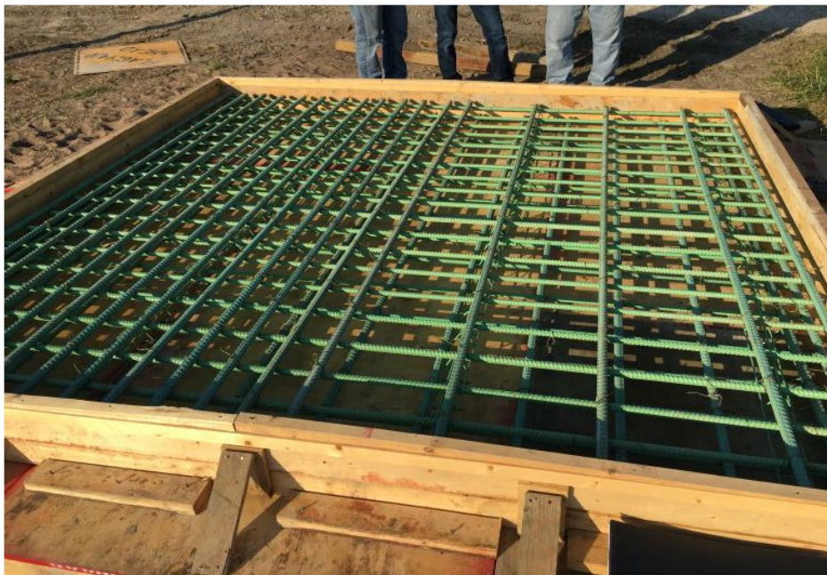
Figure 2. Mock-up slab placement with different top rebar densities of 5 x 6 in. and 10 x 6 in. that correspond to different locations along the bridge desk
