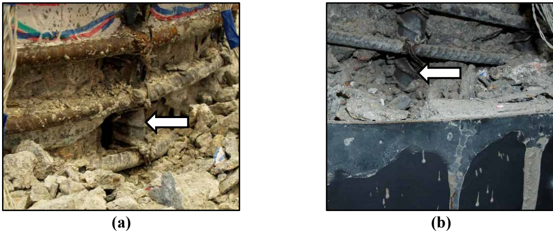
Figure 4.75: Repair #6 (a) Initiation of visible buckling of SE bar during cycle \mu_{\Delta 6}^{-ly} ; (b) Fracture of SE bar during \mu_{\Delta 6.5}^{+ly} .
