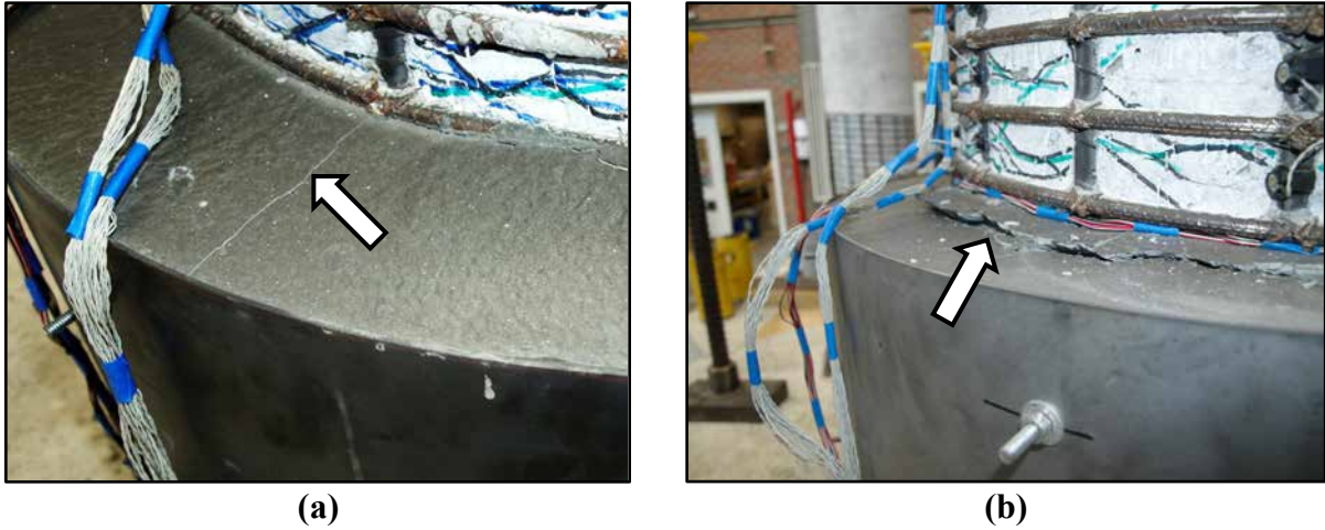
Figure 4.3: Repair #1 (a) Slight cracking on top of repair during F_y cycle; (b) progression of top surface cracking during cycle \mu_{A2}^{-2x} .
