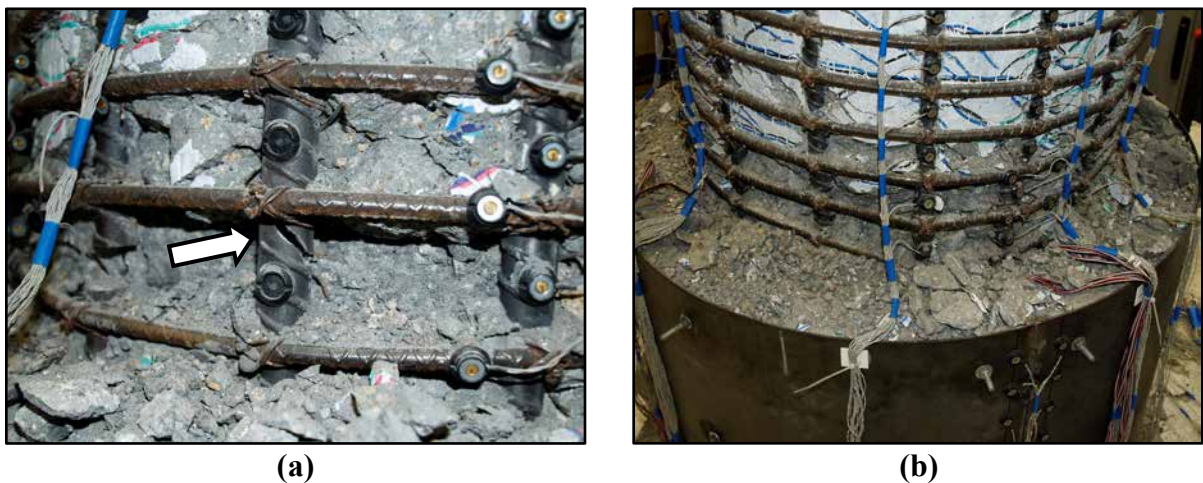
Figure 4.30: Repair #3 (a) Fracture of SSW bar during \mu_{A5}^{+2y} ; (b) Final damage state.
