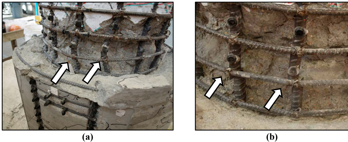
Figure 4.43: Repair #4 (a) Buckled longitudinal bars on West face; (b) Fractured longitudinal bars on South face.
