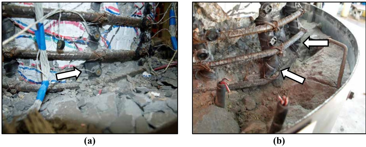
Figure 4.18: Repair #2 (a) Visible bar buckling during \mu_{\Delta 6}^{+1x} ; (b) Final damage state after multiple bar fractures during \mu_{\Delta 6}^{-1x} .
