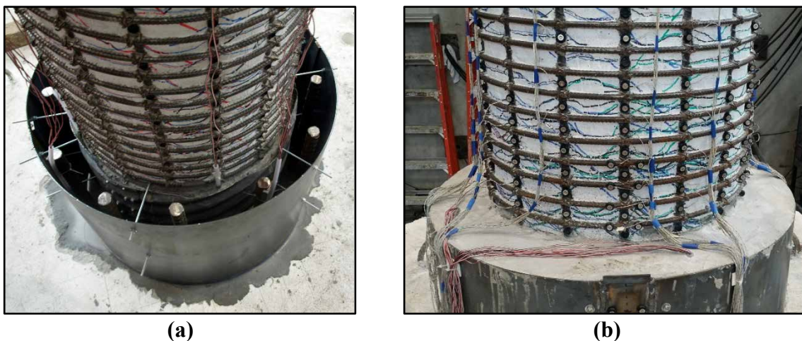
Figure 3.35: Final installation of corrugated shear key (a) before and; (b) after concrete placement.
