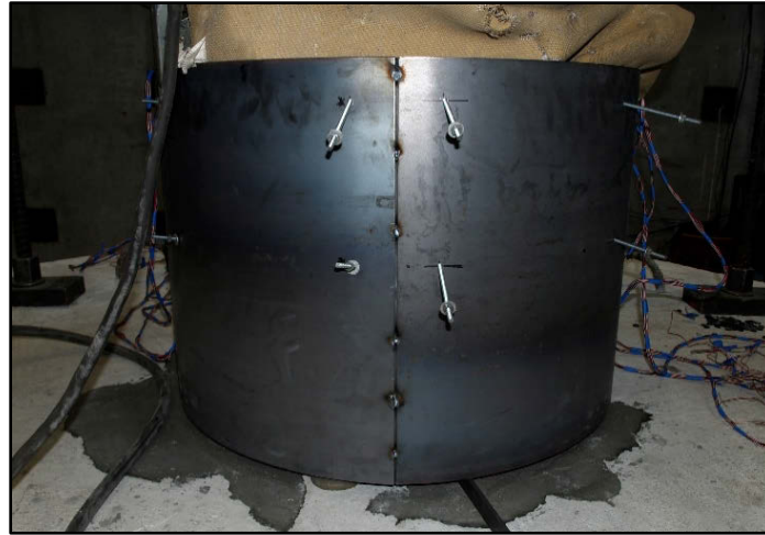
Figure 3.20: Tack welds along seam to hold sleeve and backer bar in place.
