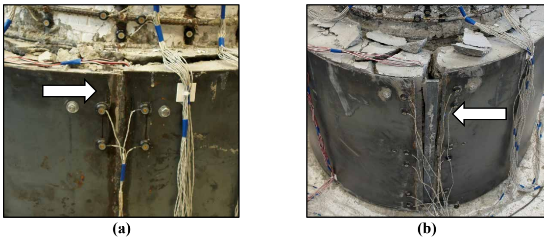
Figure 4.61: Repair #5 (a) Initiation of weld failure on South Face during cycle \mu_{\Delta 3}^{2x} ; (b) Complete weld failure on North Face during cycle \mu_{\Delta 4}^{-2y} .
