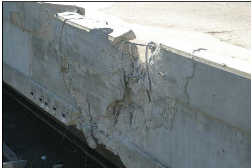
Figure 17. Bridge Rail T501 at Location A after Test B4.
