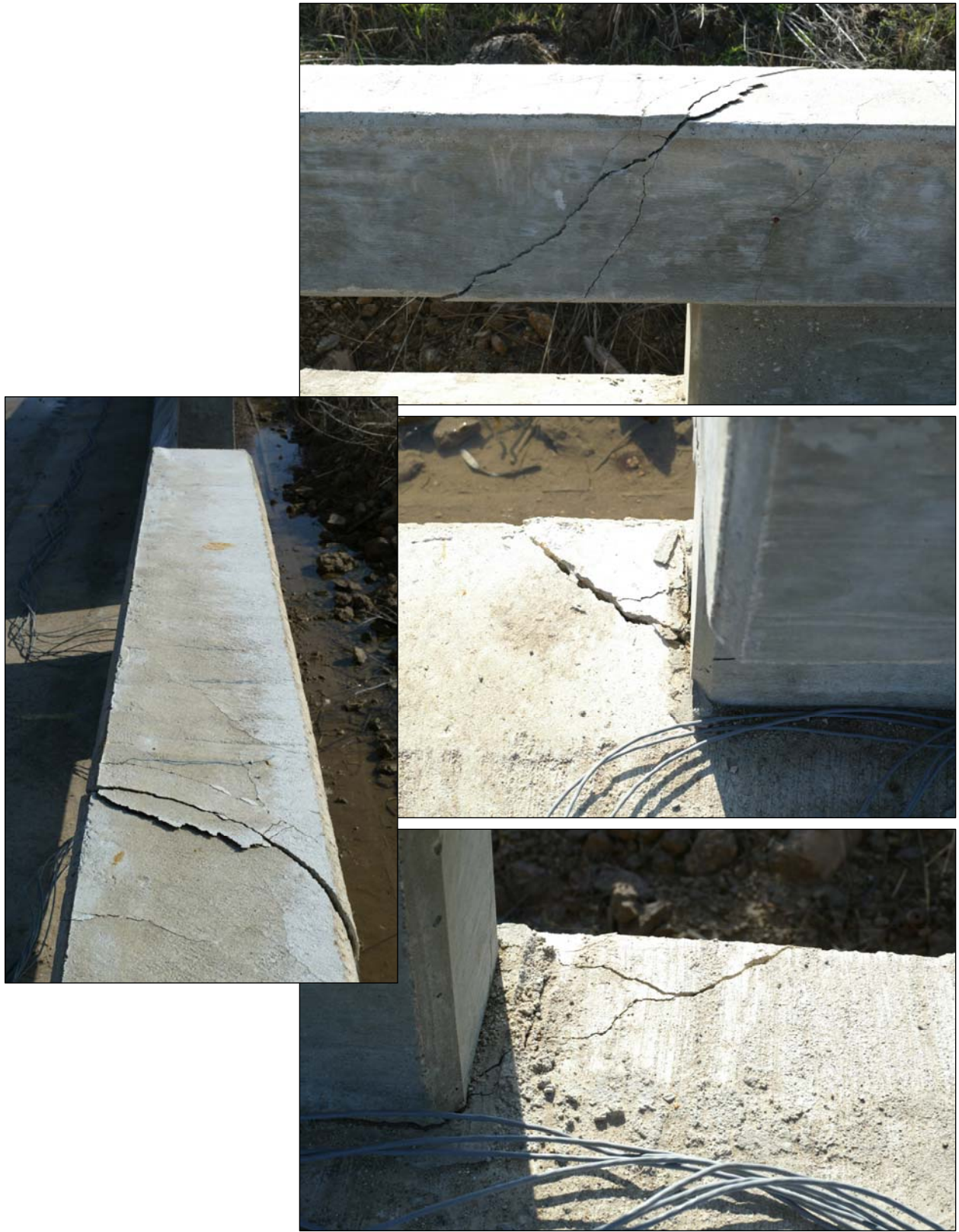
Figure 15. Bridge Rail T203 at Location D after Test B2.
