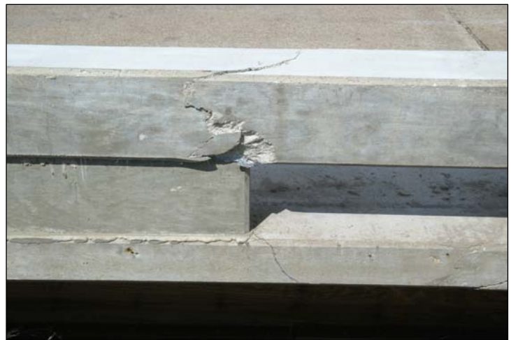
Figure 14. Bridge Rail T203 at Location F after Test B1.
