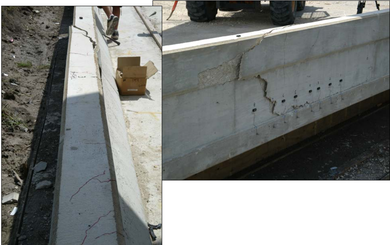
Figure 9. Bridge Rail T501 at Location A after Test S4.
