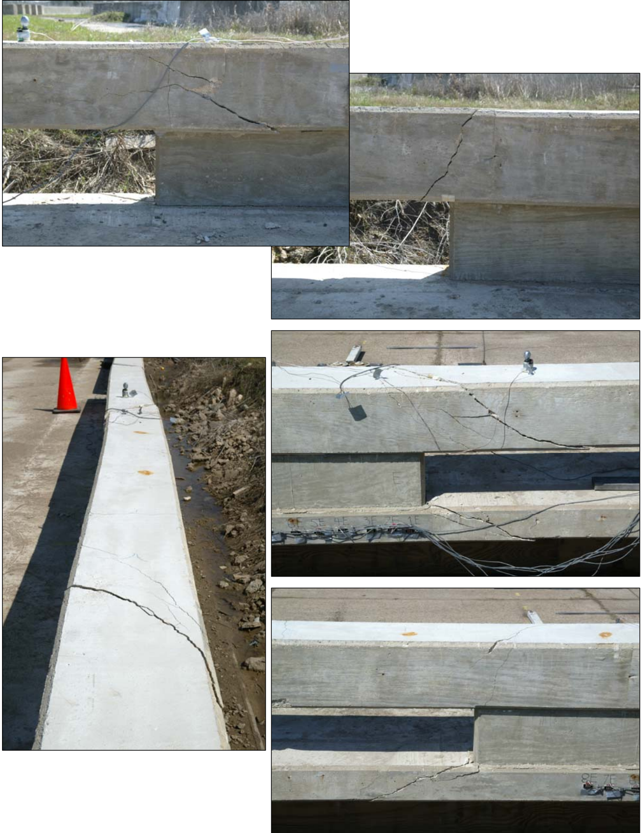
Figure 16. Bridge Rail T203 at Location E after Test B3.
