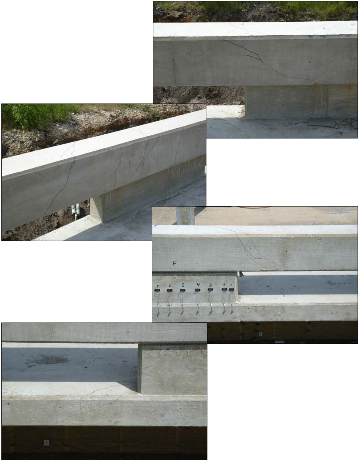
Figure 6. Bridge Rail T203 at Location F after Test S1.
