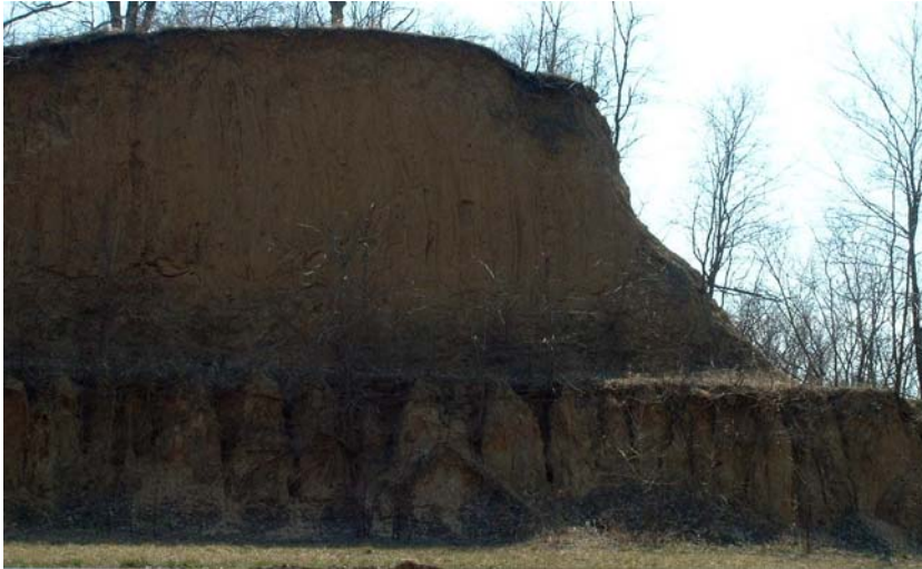
Figure 2.3: Vertical cuts formed by erosion in bluff along Highway 210 in North Kansas City, Missouri
