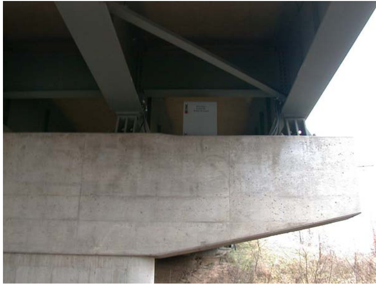
Figure 4.9. Photograph of DAS enclosure on Pier 2.
