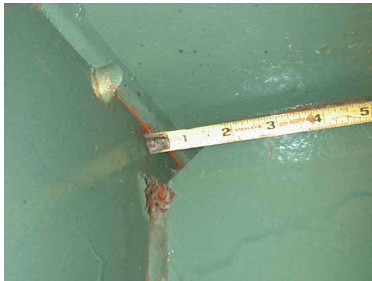
Figure 2.7. Photograph of typical web gap.
