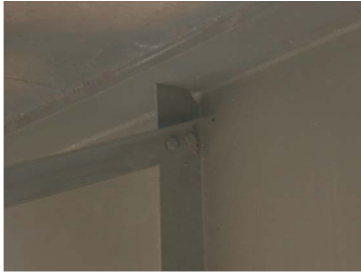
Figure 4.6. Photograph of typical web gap.
