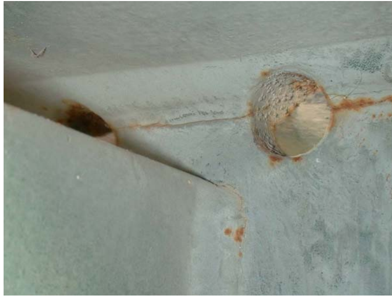
Figure 3.11. Typical drilled hole retrofit in web with continued cracking.
