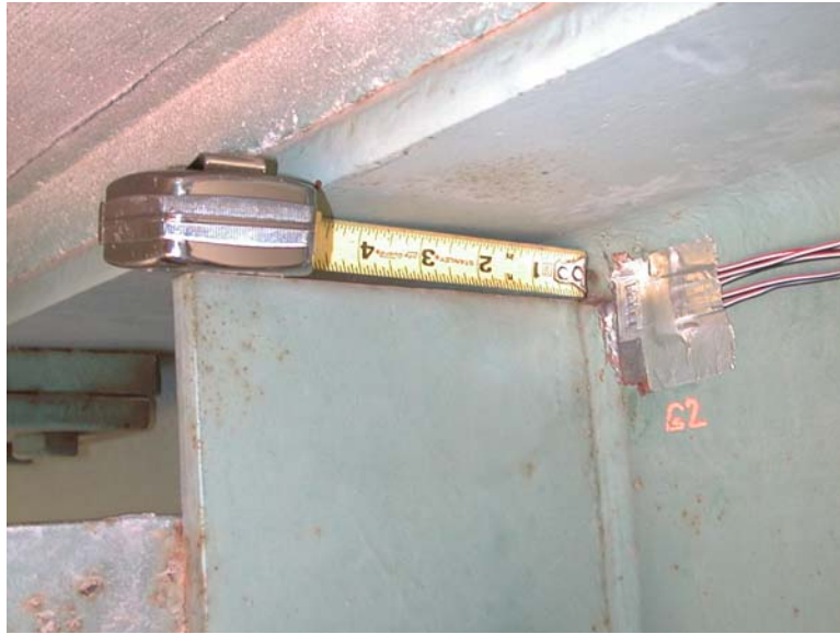
Figure 3.7. Typical web gap in negative moment region.
