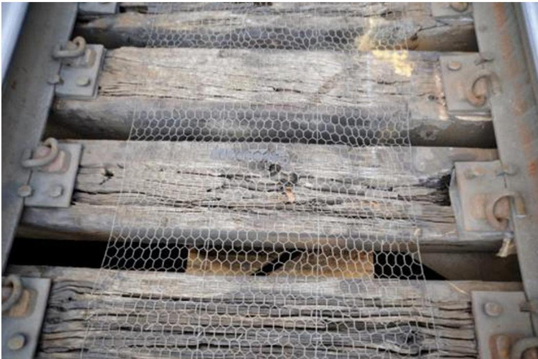
Figure 46 - Deteriorated railway ties at the location of high settlement..
