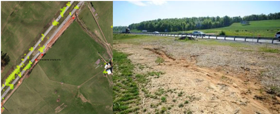
Figure 48 - TS points along I-81 (left) and surface erosion at the TS point locations (right).
