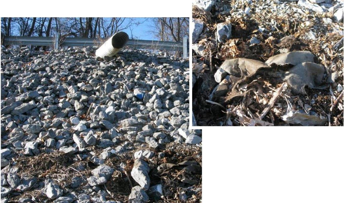
Figure 40 - Site Conditions and Deterioration at Rock Buttress.
