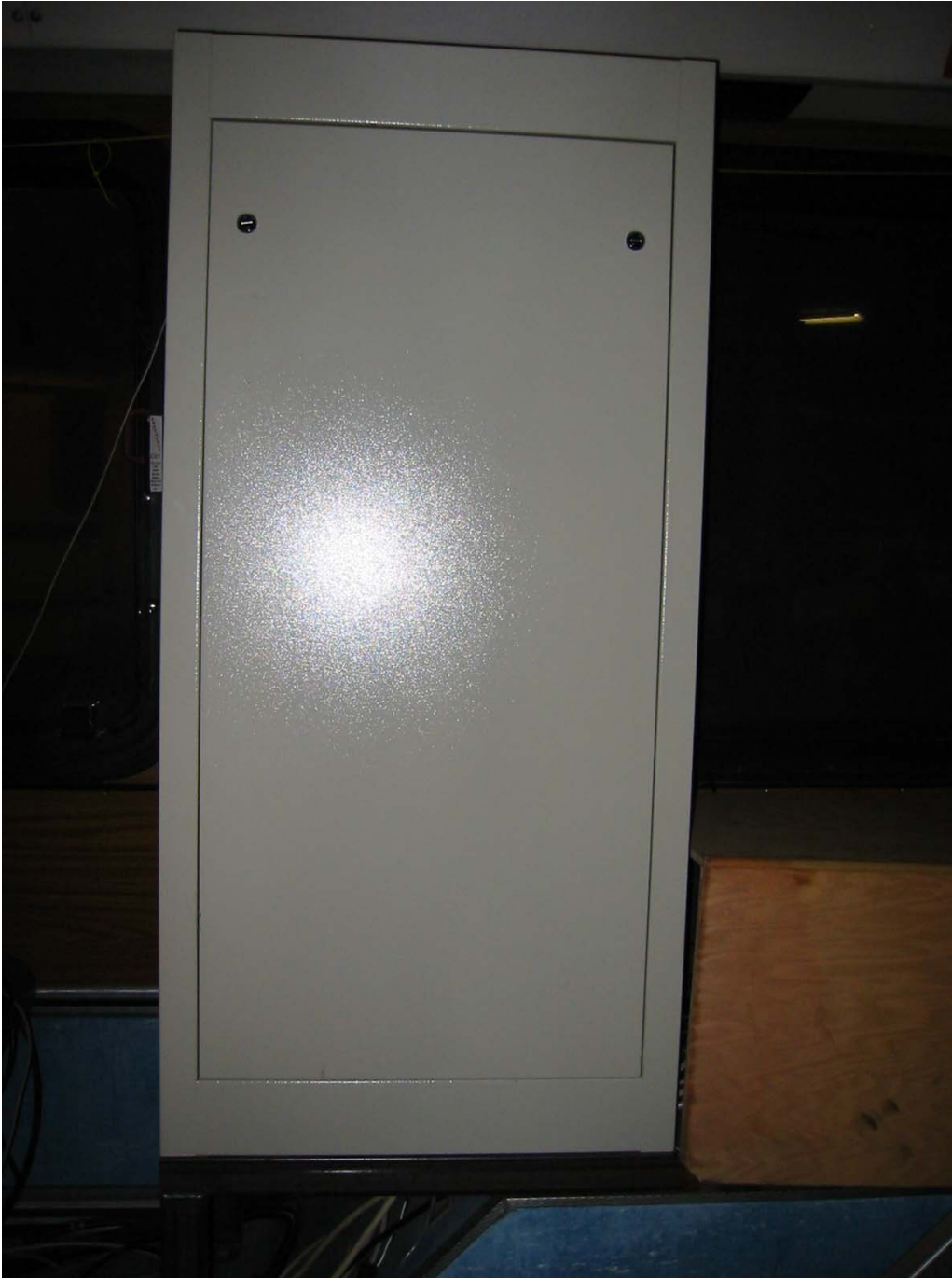
Picture 15. Equipment cabinet on Technobus research vehicle. Cabinet sits over left front wheel on a custom steel frame where the forward most center facing seats are typically mounted. Cabinet is approximately four feet (1.2 m) tall. Oak veneered box to cabinet left covers AC inverter, battery equalizer (splits 24 VDC to 12VDC), and amplifier for servo motor.
