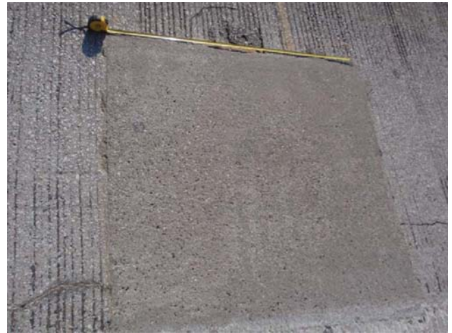
Figure C.9 Patch area originally repaired with SET 45 Regular material which has been since replaced.
