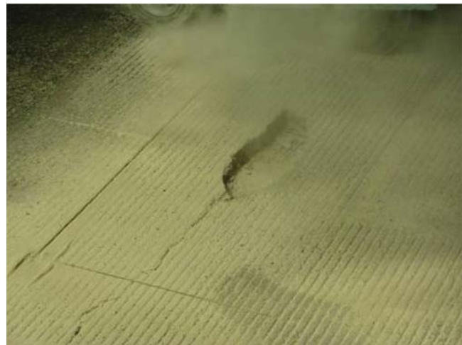
Figure 5.5 Distress III: pothole (spall) in the existing concrete (northbound direction).
