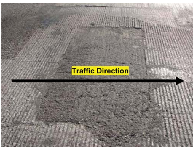
Figure B.5 SikaQuick-2500 patch-I.
