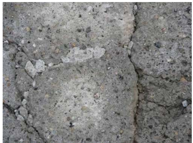
Figure 8.3 Appearance of the SET 45-R material in the deteriorated patch.
