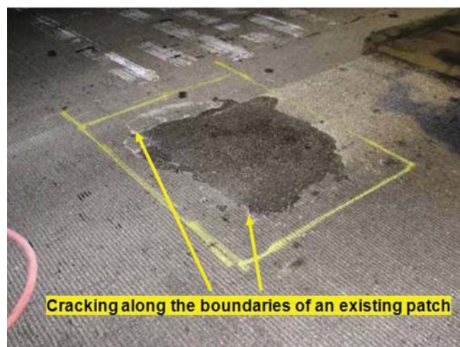
Figure 5.3 Distress I: cracking along boundaries of an existing patch (southbound direction).
