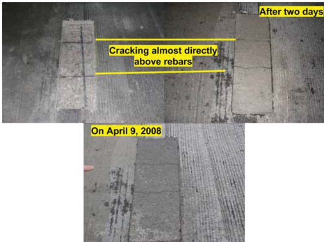
Figure A.9 SikaQuick-2500 patch-II: overview.
