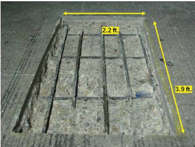
Figure 5.26 FX-928: patch area-I.
