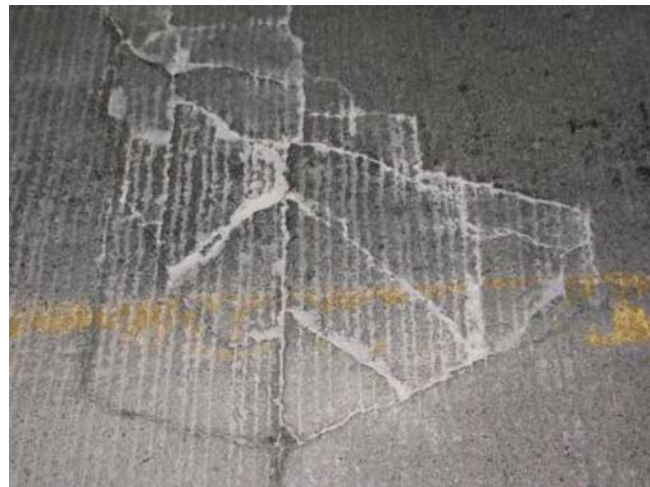
Figure 5.4 Distress II: severe cracking of existing concrete (northbound direction).
