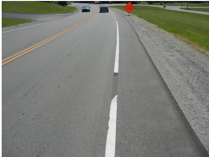
Franklin County; KY 420; Inlaid Tape; Snowplow Damage
