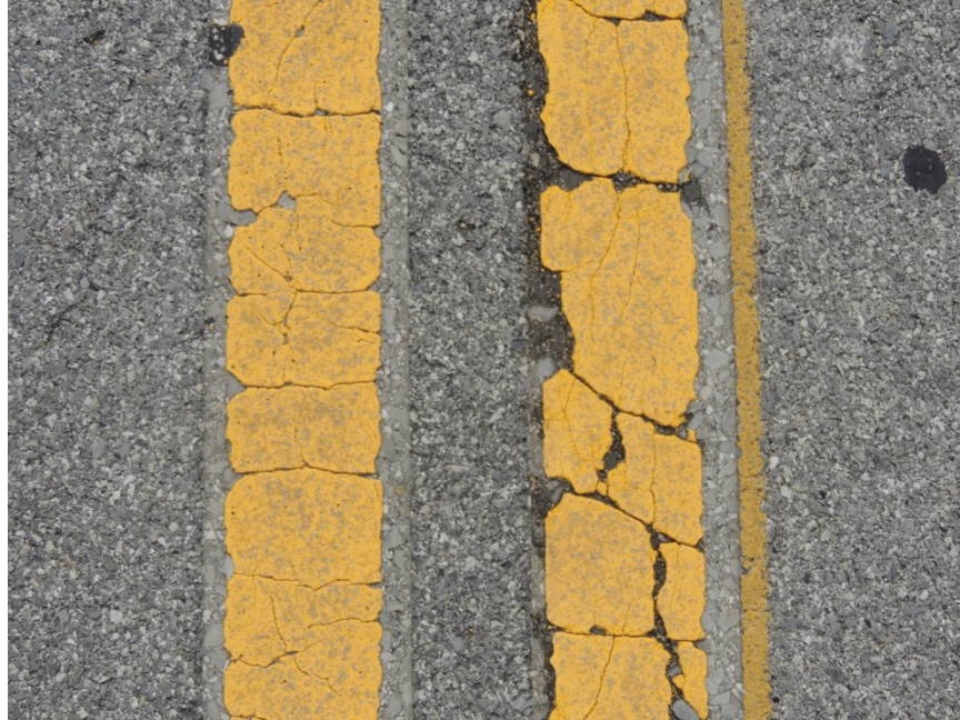
Warren County; KY 234; Cracking of Thermoplastic Material
