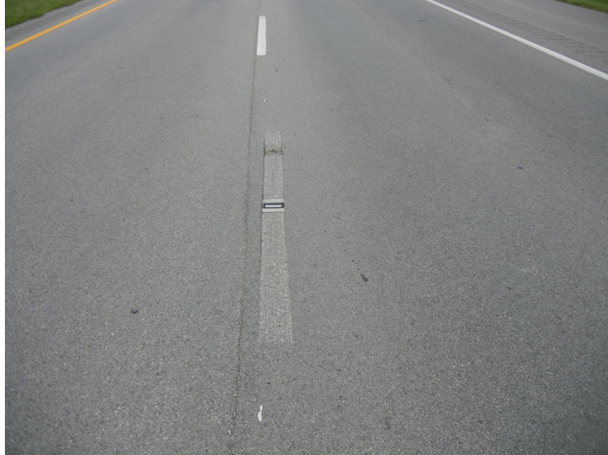
Mercer County; US 127; Recessed Marker; Lenses Missing
