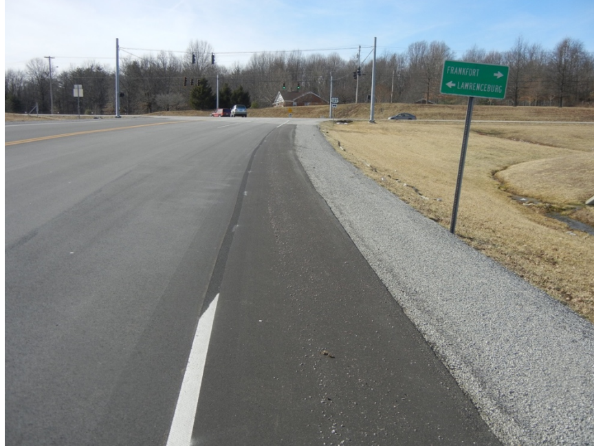
Franklin County; KY 420; Inlaid Tape; Snowplow Damage
