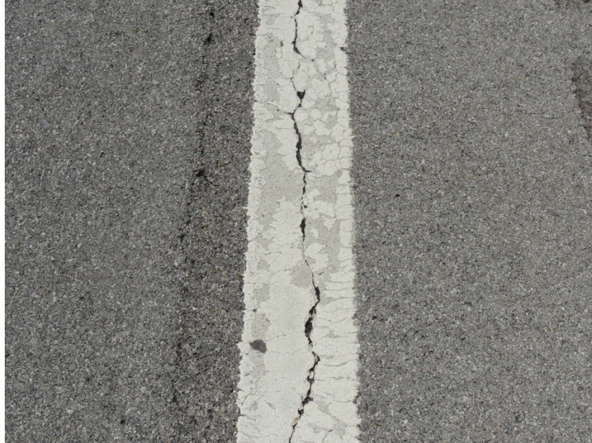
Simpson County; I-65; Spray Thermoplastic; Snowplow Damage
