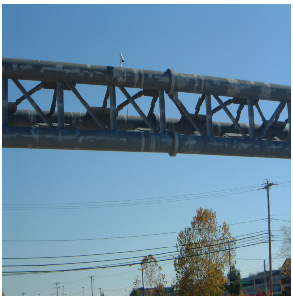
VID Camera mounted on full-span structure
