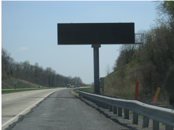
VMS – Center-mount roadside structure
