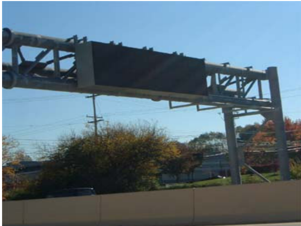
VMS – Mounted over road on full-span structure
