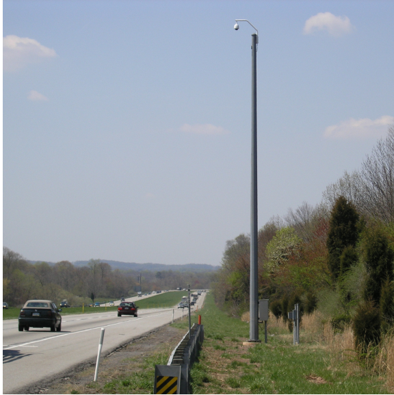
Typical CCTV installation – 50-foot pole
