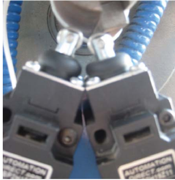
Figure 3.6 Ending position limit switch engaged.
