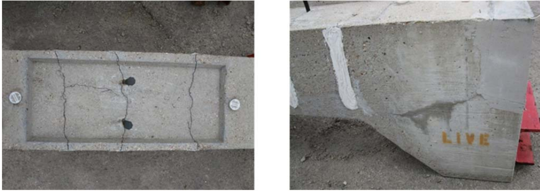
Figure 5.22: Specimen 1.2 Top Surface (Left) and Leakage at Live End Corbel Crack (Right)
