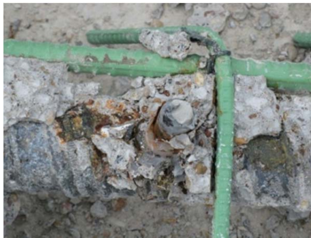
Figure 5.30: Specimen 2.2, Corrosion Staining Under North Grout Vein
