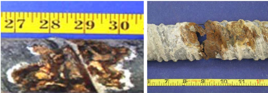
Figure 6.20: Typical Galvanized Steel Duct from Project 0-14058 (Left) and Project 0-4562 (Right)
