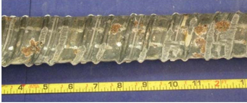
Figure 5.16: Specimen T.2, Corrosion Along Gouges on Bottom Half of North Duct
