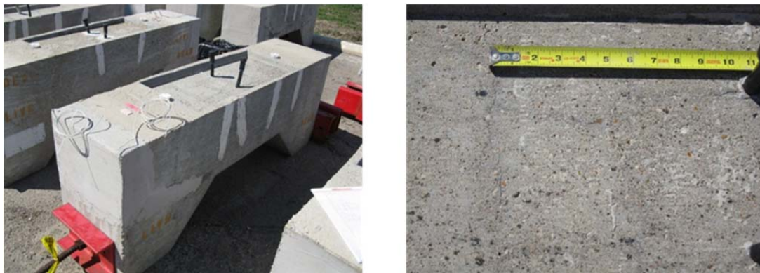
Figure 5.59: Specimen 3.4 Overall (Left) and Discoloration around Surface Cracks (Right)
