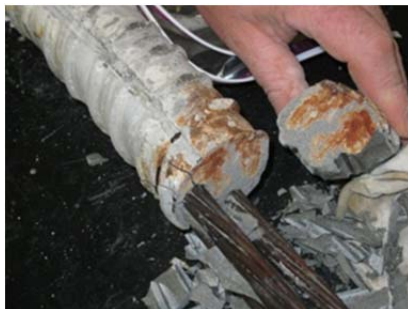
Figure 5.24: Corrosion Staining Within South Grout
