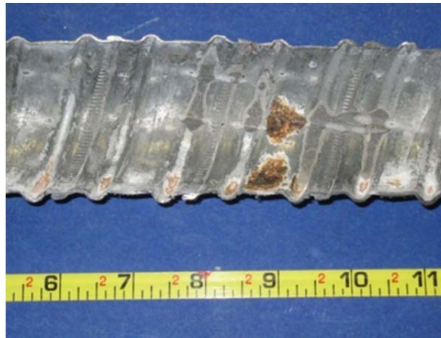
Figure 5.9: Specimen T.1, Corrosion Along Gouges on Bottom Half of North Duct
