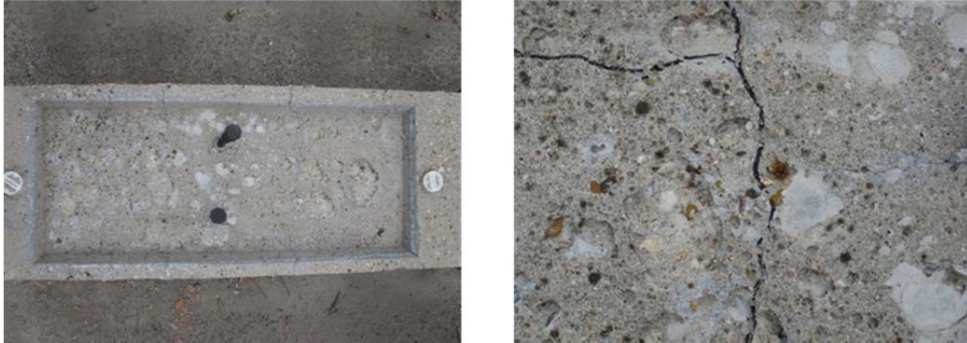
Figure 5.41: Specimen 3.1 Top Surface (Left) and Corroded Wire Tie at Top Surface (Right)
