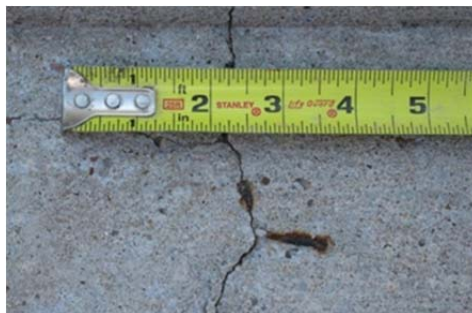
Figure 5.35: Specimen 2.4, Corroded Wire Tie at Top Surface
