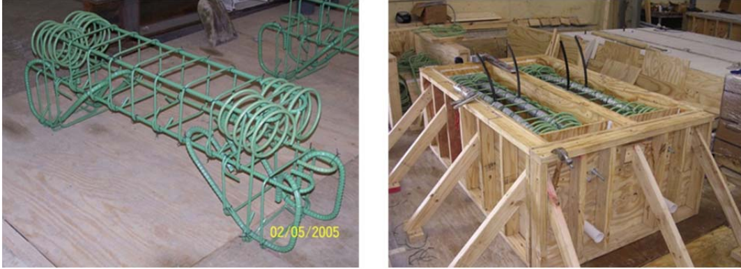
Figure 2.5: Epoxy-Coated Rebar Cage (Left) and Completed Reinforcement Cage with Ducts in Formwork (Right) 7
