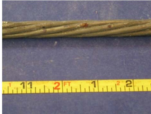
Figure 5.17: Specimen T.2, North Duct Strand Showing Pitting Near Midspan
