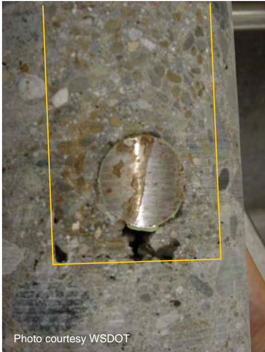
Figure A-69. Poor consolidation.
