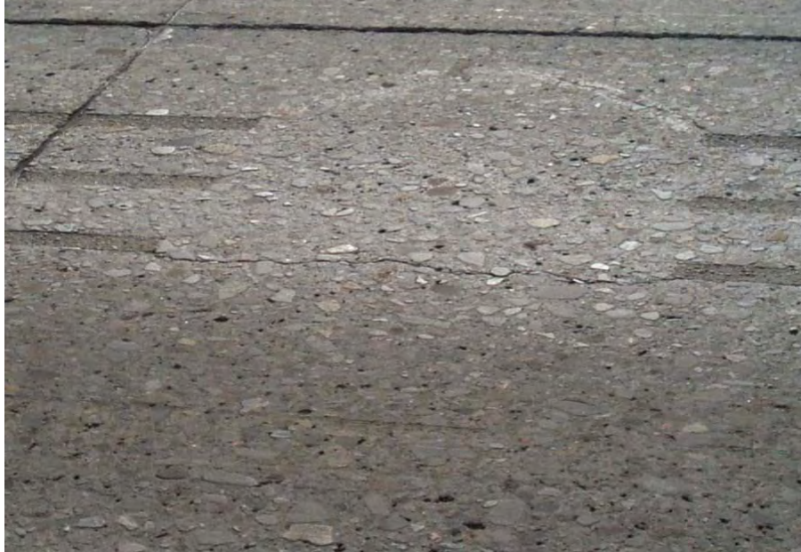
Figure 197 Longitudinal cracking after dowel bar retrofit.
