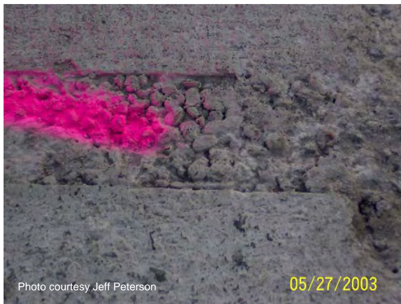
Figure A-47. Insufficient consolidation of patching material.
