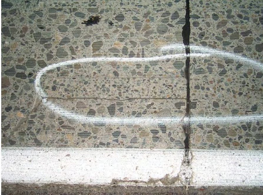
Figure 207 Debonding of patching material.
