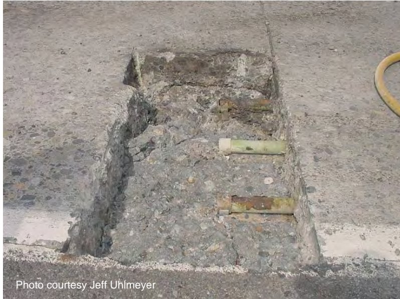
Figure A-60. Corroded epoxy coated dowel bars.
