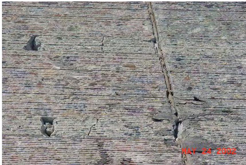
Figure 127 Shrinkage cracking and spalling State Route 8 (Glauz et al., 2002b).
