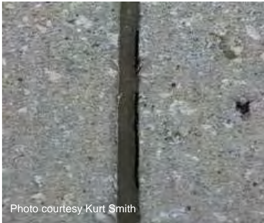
(a) Adhesive failure.
