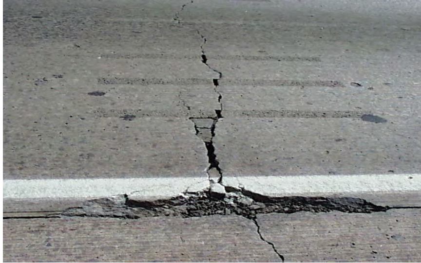
Figure 136 Spalling of dowel bar retrofitted transverse crack.
