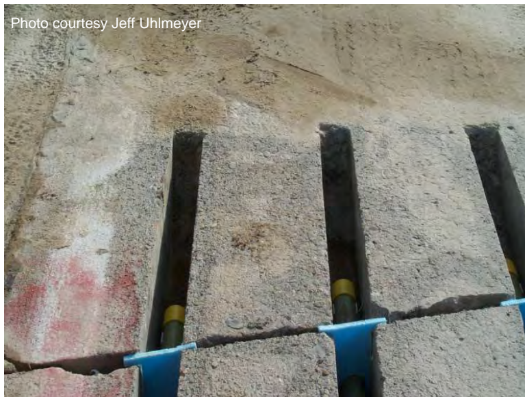
Figure A-49. Debris should be cleared to a sufficient distance to prevent intrusion.
