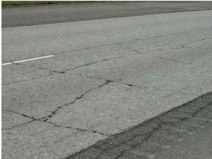
Figure 154 Test section – multi-cracked slab.
