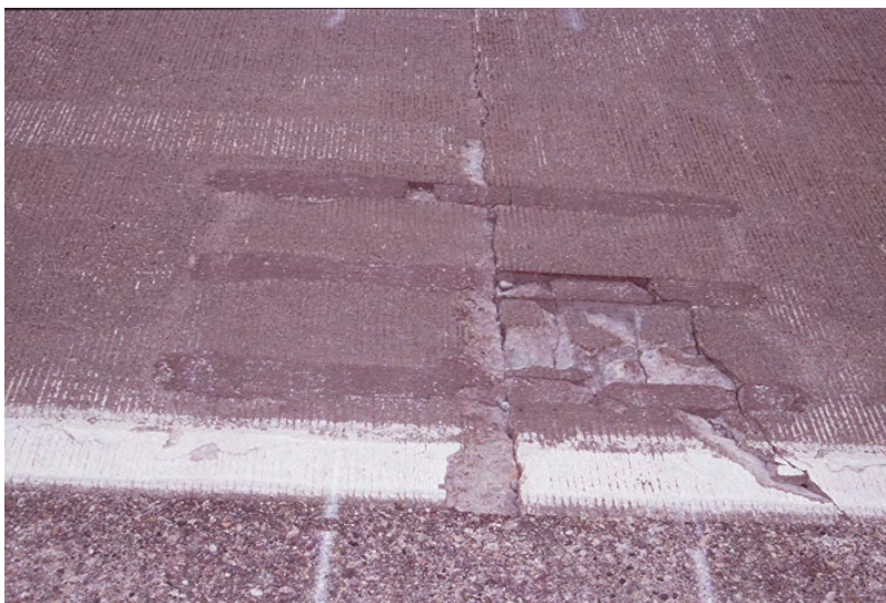
Figure 134 Cracking between dowel bar slots.
