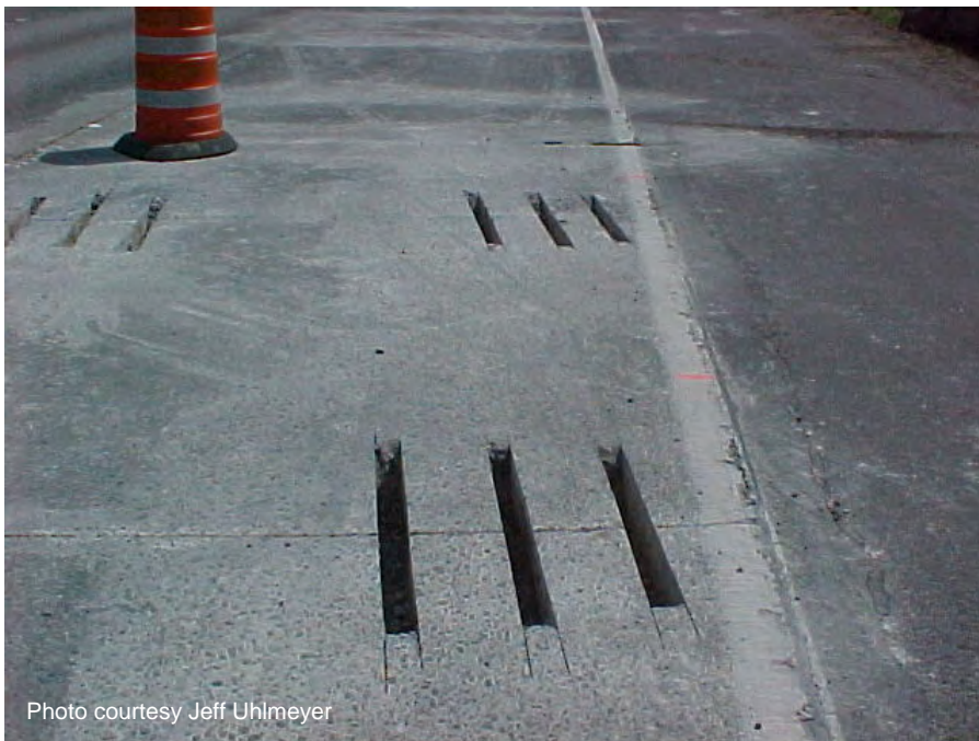
Figure A-15. Dowel bar slots incorrectly cut on skewed joints.
