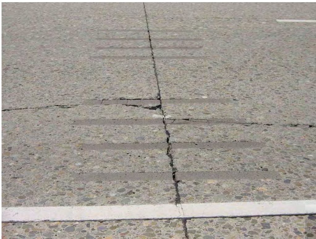
Figure A-20. Failure of dowel bar slot placed over existing longitudinal crack.
