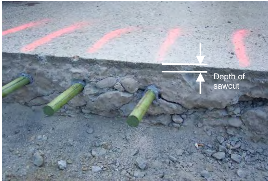
Figure 236 Panel not sawcut full-depth.
