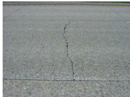
b. Transverse cracking
