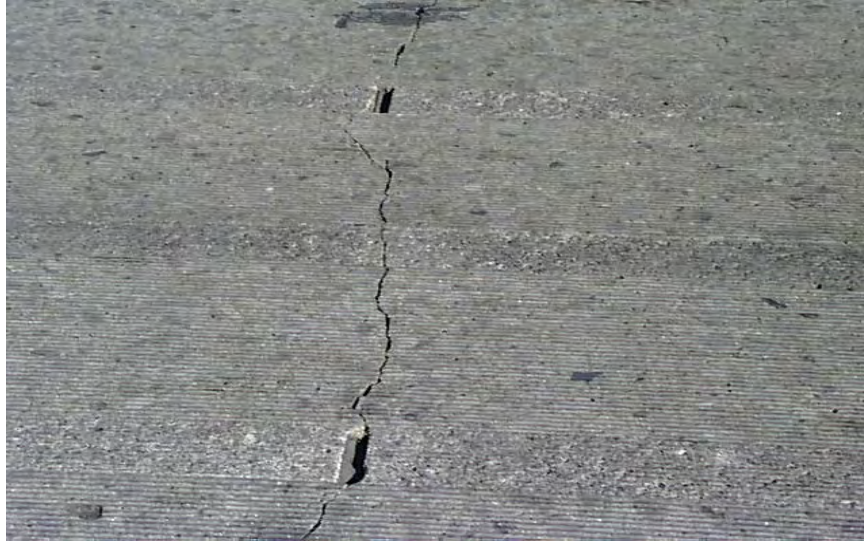
Figure 135 Minor spalling between foam core board and transverse crack.
