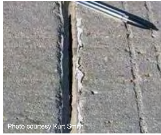
(b) Cohesive failure.
