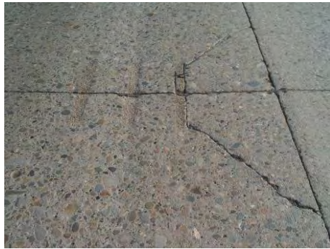
(e) 45-degree cracking.
