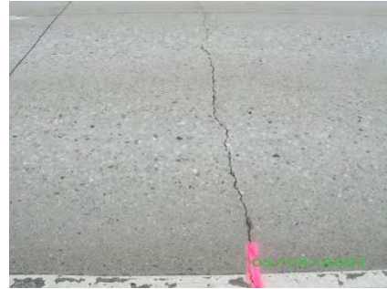
(b) Transverse cracking.
