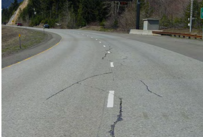
Figure 28 Longitudinal cracking caused by failed tape joint.
