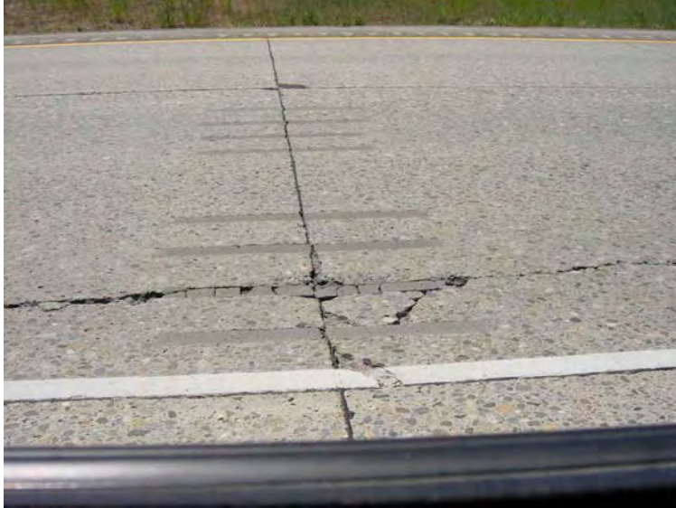
Figure 225 Existing longitudinal crack at dowel bar retrofit slot.
