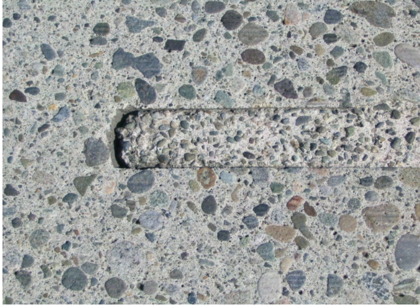
Figure A-44. Patching material bond failure.
