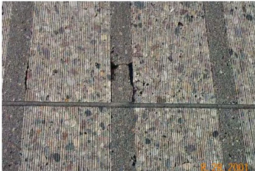
Figure 121 Typical distress in Patchroc 10-60 (Dunn et al., 1998).
