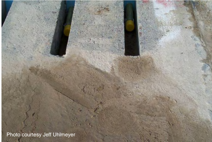
Figure 124 Debris left adjacent to dowel bar slots.
