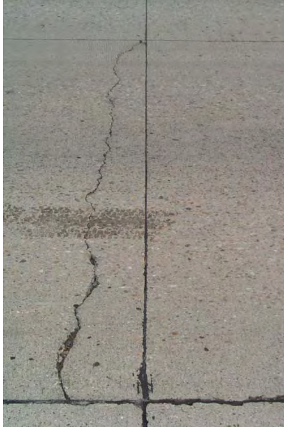
Figure A-22. Transverse crack is functioning as the working joint.
