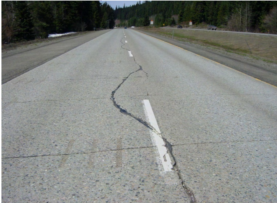
Figure 179 Failed longitudinal tape resulting in longitudinal cracking.
