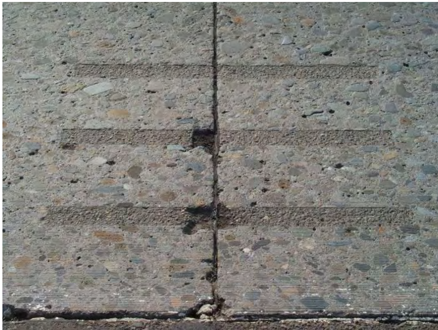
Figure 204 Spalling of patching material.
