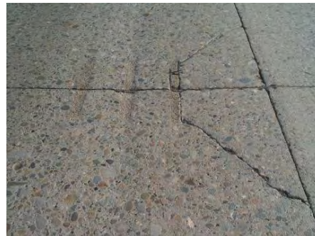
d. 45-degree cracking
