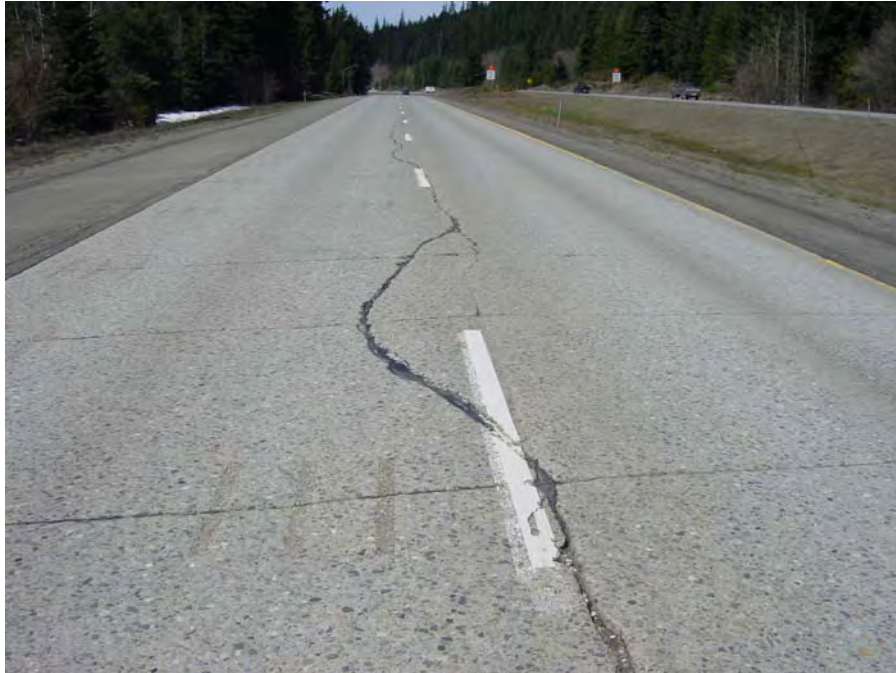
Figure A-19. Left wheelpath dowel bar slots not installed to avoid existing longitudinal crack.
