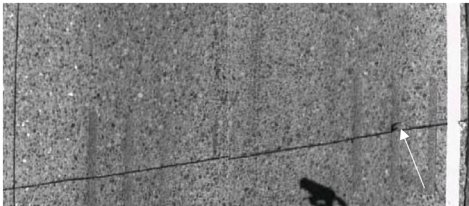
Figure E-24 Low severity spalling within dowel bar slot.
