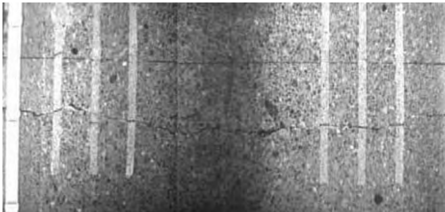
Figure E-6 Dowel bar retrofitted transverse crack and joint.
