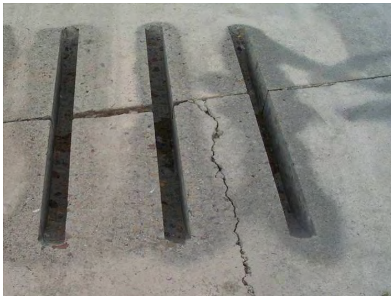
Figure A-18. Dowel bar slots aligned to miss an existing longitudinal crack.
