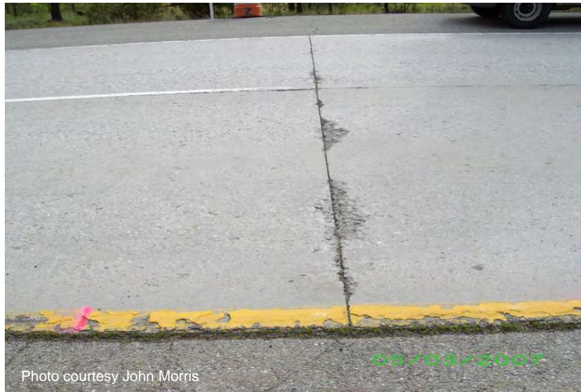
Figure 18 Spalling at a transverse joint.
