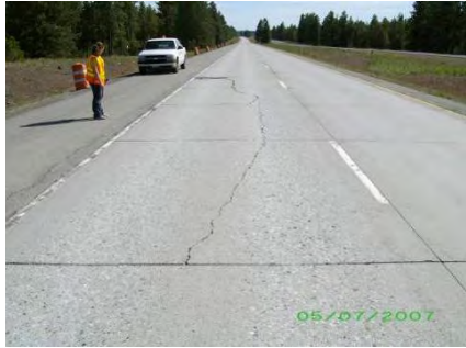
(a) Longitudinal cracking.
