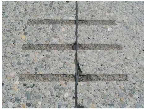
(a) Dowel bar slot spalling.
