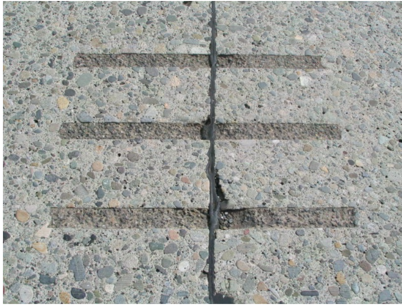
Figure A-46. Spalling of patching material.
