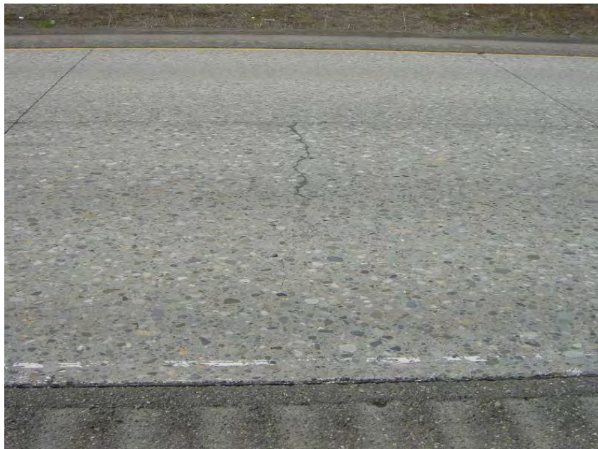
Figure 195 Transverse cracking after dowel bar retrofit.
