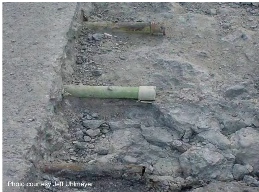
Figure A-59. Corroded epoxy coated dowel bars.
