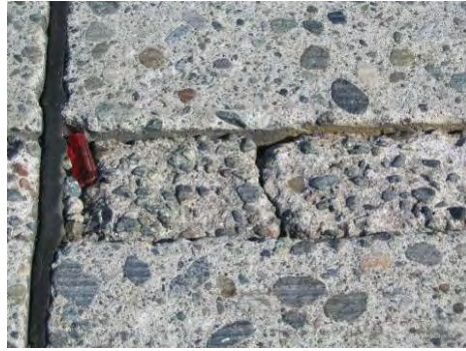
(b) Dowel bar slot cracking.
