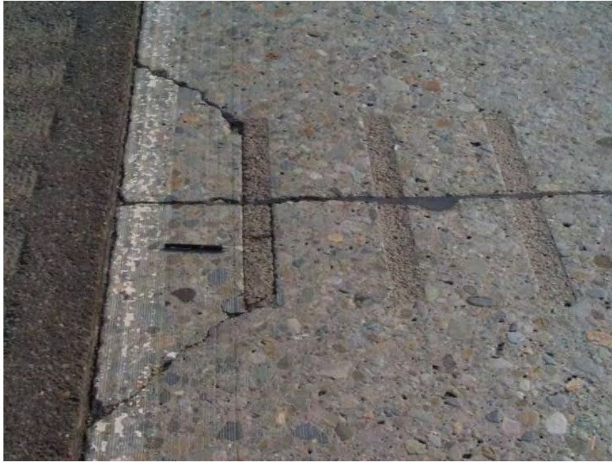
Figure A-16. Dowel bar slot cut and/or chipped to deep.
