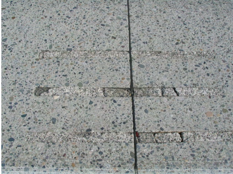
Figure 200 Patching material cracking.
