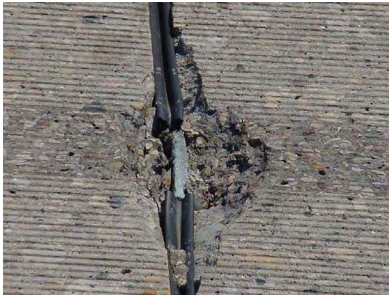
Figure 122 Mortar deterioration and spalling (Wilson et al., 2002).
