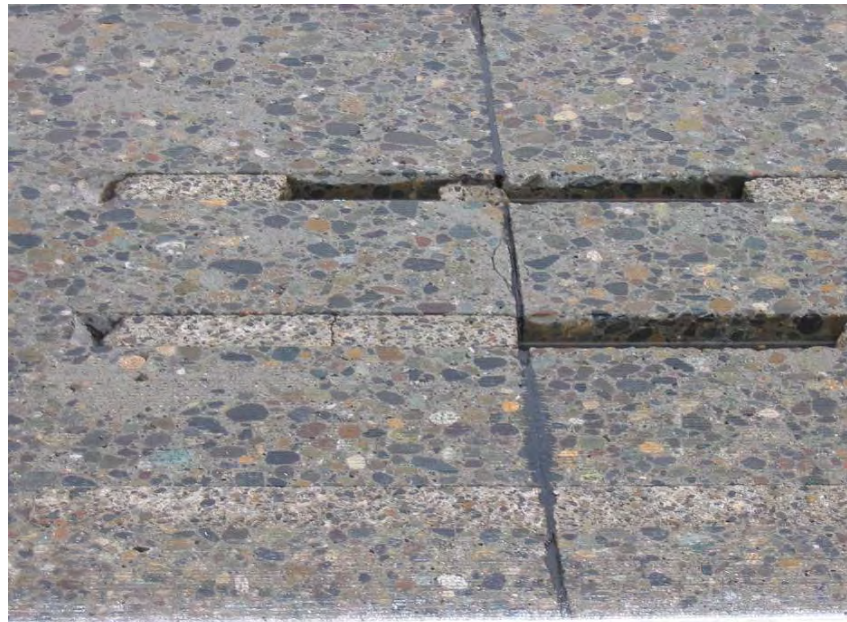
Figure A-45. Patching material bond failure.
