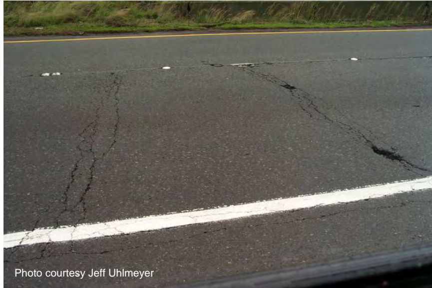
Figure 106 Reflection cracking (I-5 Centralia vicinity).
