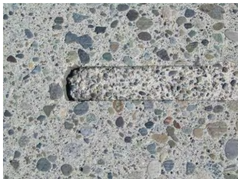
(c) Dowel bar slot debonding.
