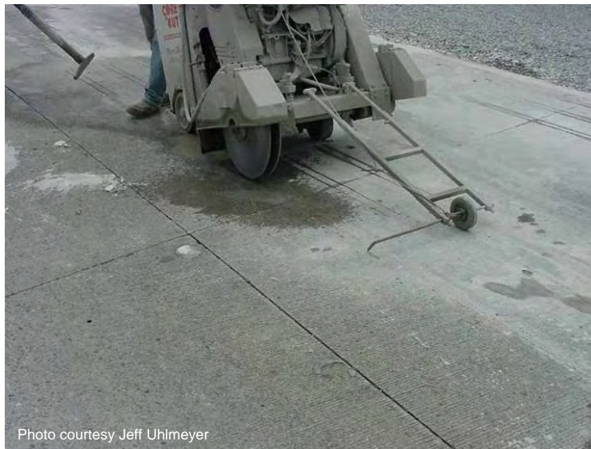
Figure A-12. Cutting equipment for one dowel bar slot at a time.
