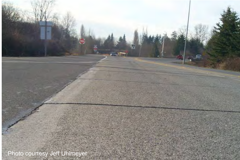
Figure 19 Transverse joint faulting.
