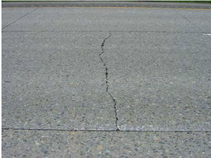
Figure 152 Test section – transverse cracking.
