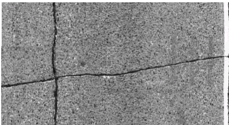
Figure 227 Dowel bar retrofit eliminated in left wheelpath to avoid longitudinal crack.
