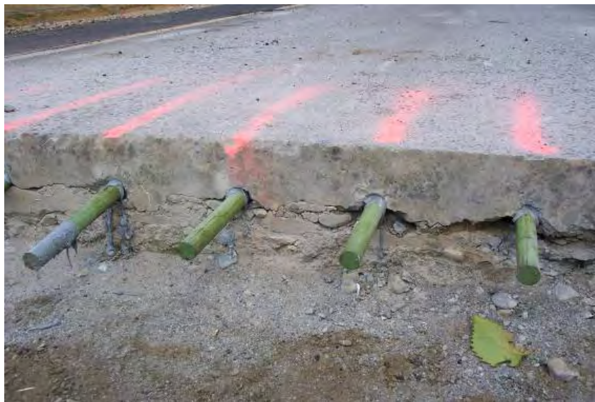
Figure 237 Spalling of concrete slab during drilling for dowel bars.
