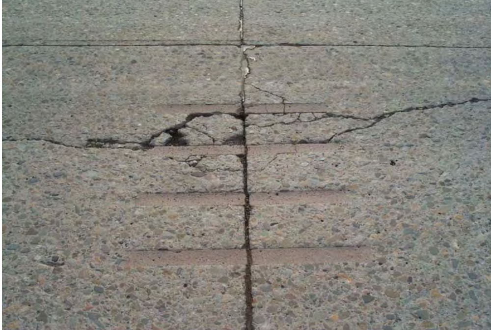
Figure A-21. Failure of dowel bar slot placed over existing longitudinal crack.
