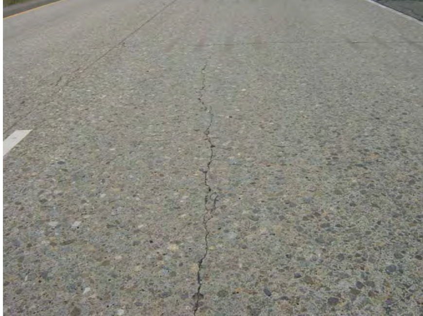
Figure 153 Test section – longitudinal cracking.
