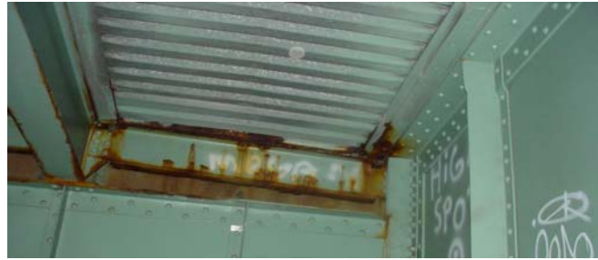
Figure 5. Localized Rusting Near Expansion Joint
