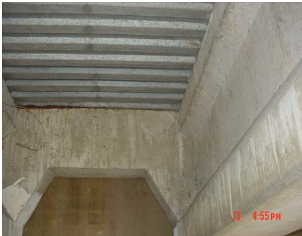
Figure 1. 40-year old SIPMF on Precast Girders. Note Localized Rusting Near Expansion Joint
