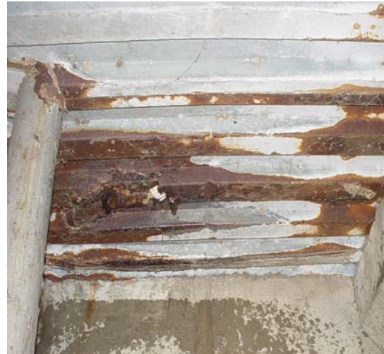
Figure 2. Localized Rusting Near a Scupper Hole and Drain Pipe
