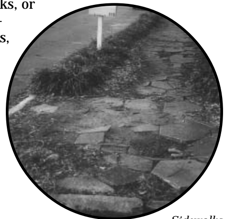
Sidewalks with cracked, uneven pavement and no ramp make it difficult for strollers and wheelchairs to cross.
