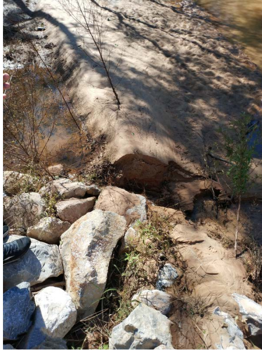
Figure 5- 47: Aggradation signs on the east side of Soapstone Branch, downstream from temporary steel bridge
