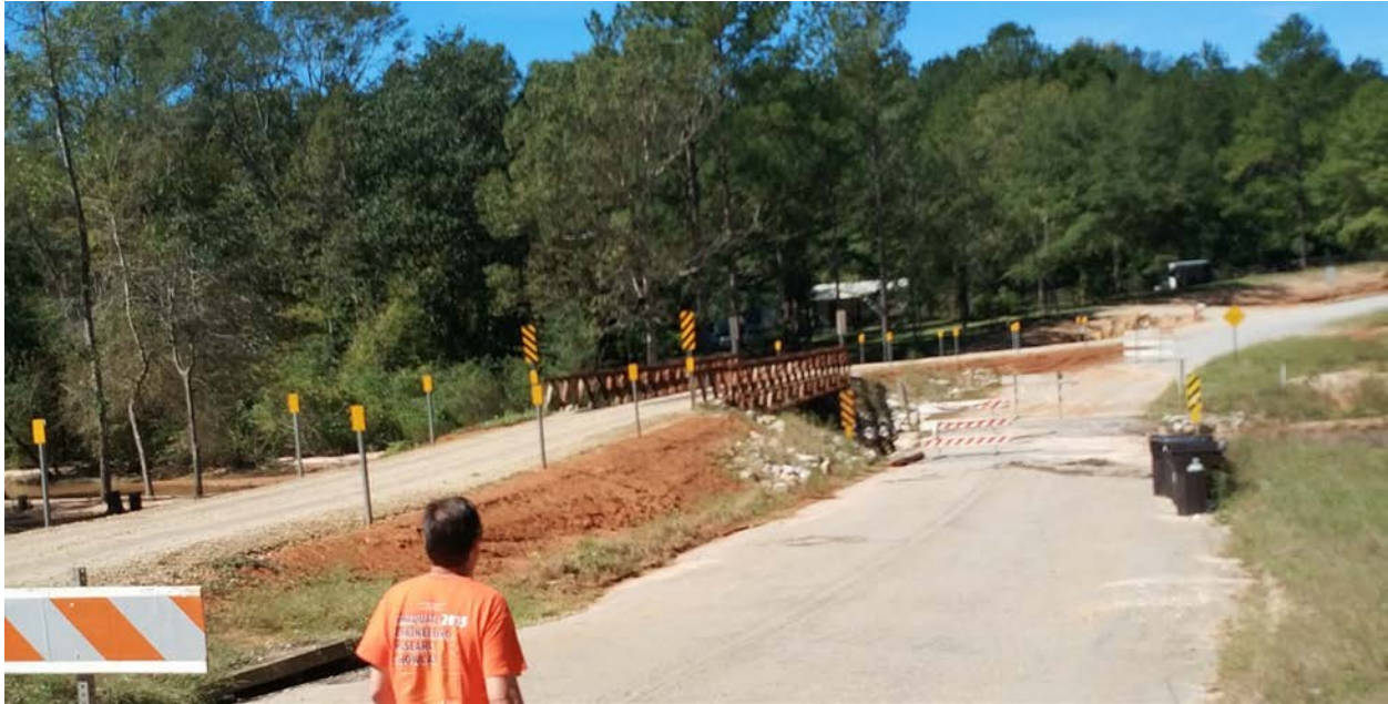
Figure 5- 45: Temporary steel bridge placed in parallel to the old Dean Road Bridge over Soapstone Branch.
