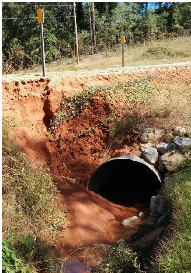
Figure 5- 48: Surface erosion in the eastern embankment and erosion created by stormwater flows from Dean Road, creating slope failures immediately upstream from the temporary steel bridge.
