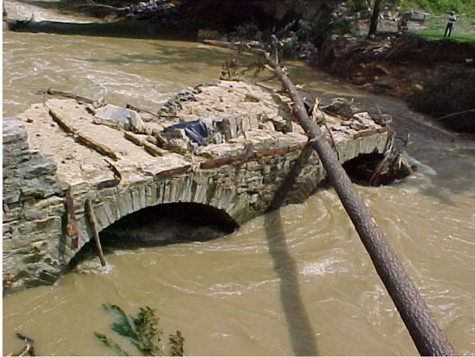
The remains of the Falling Creek Bridge on the afternoon of August 31, 2004. For perspective, note the size of the man in the upper right corner.
