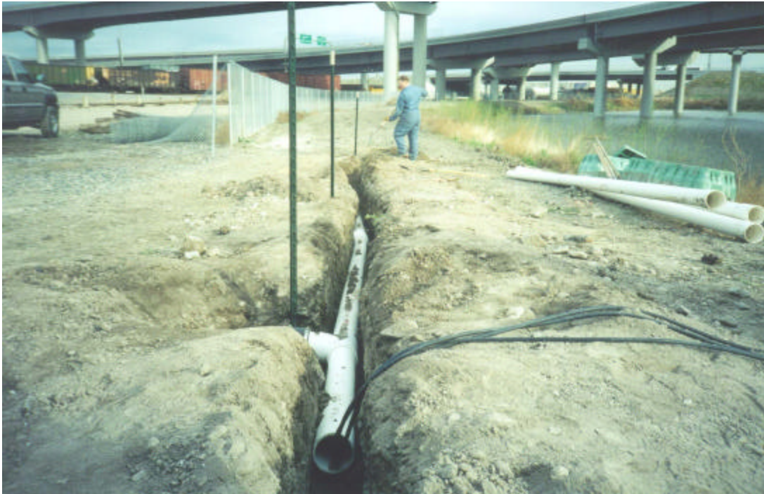
Figure 4.3. Partially installed conduit with three electrical cables threaded through pipes; note fence posts driven to mark wellhead locations
