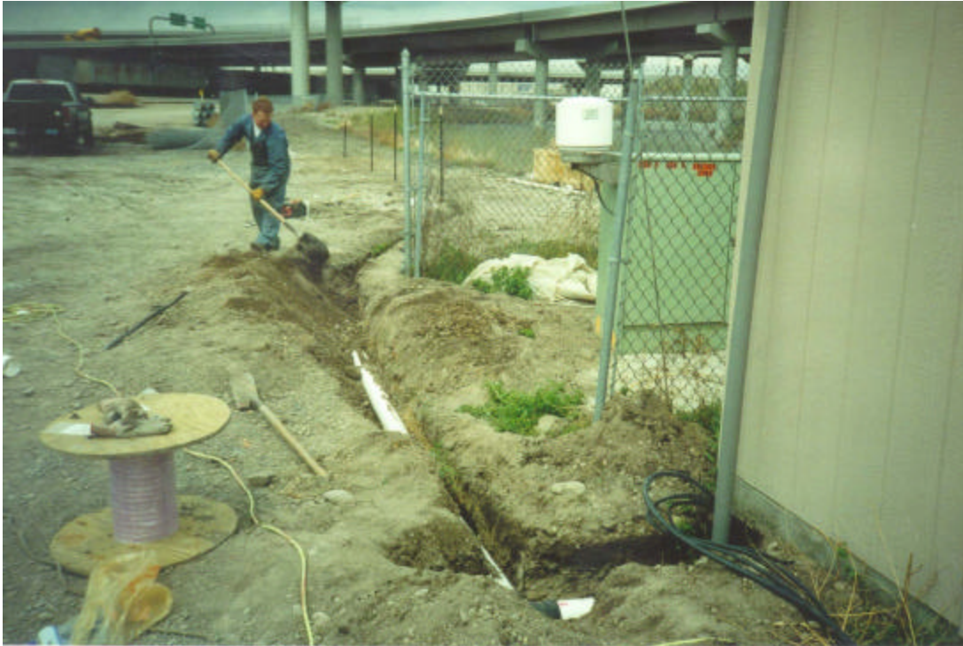
Figure 4.4. White electrical conduit, being covered, placed extended to the instrument shed foundation; a gray, external-grade electrical conduit riser is leaning against the shed; the electrical cables lying on ground surface have yet be pulled through the gray conduit
