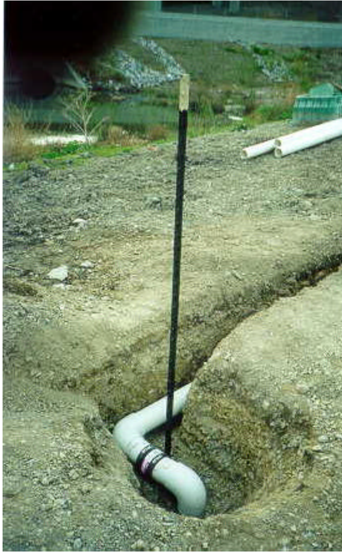
Figure 4.2. PVC pipe electrical conduit extending from the top of the 25-ft (7.6-m) casing and to the trench leading to the instrument shed; note that a steel fence post has been driven near the conduit to mark the approximate location of the wellhead
