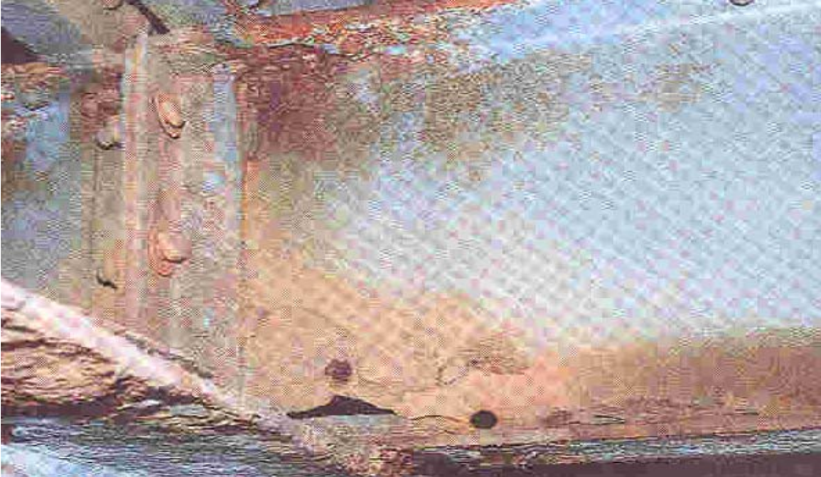
Figure 1.2 Deterioration near steel beam end (photo taken by MDOT bridge inspector)
