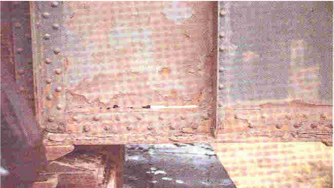
Figure 1.3 Deterioration near steel beam end (photo taken by MDOT bridge inspector)
