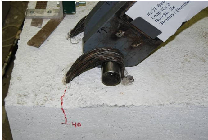
Figure 1: First Cracking (Stage 1)
