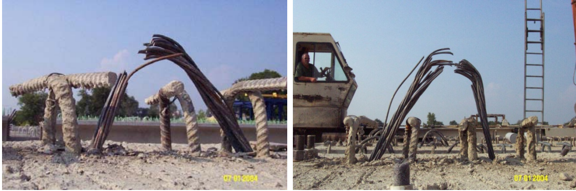
Figure 1. Lifting loop strand rupture failures in field (courtesy of IDOT).
