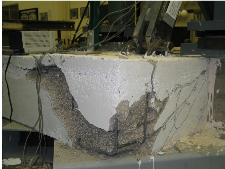
Figure 20. Two lifting loops in a corner of a deck beam demonstrating a “cone” separation, concrete intact surround loop.
